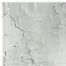
Peeling lead paint
