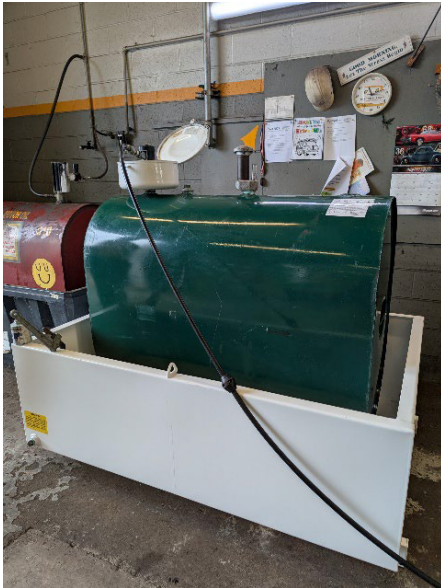
Photo: A green fuel storage tank installed in a white secondary-containment basin inside a garage bay.
