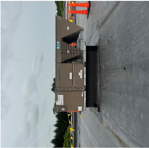
Photo: A large brown rooftop HVAC unit staged outdoors on pavement, marked off with orange safety cones.
