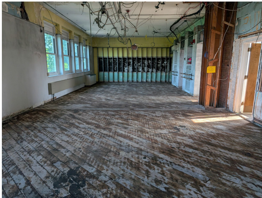
Photo: A large, gutted room with damaged wood flooring, stripped walls, and electrical wiring hanging exposed from the ceiling, with sunlight coming through windows on the left.
