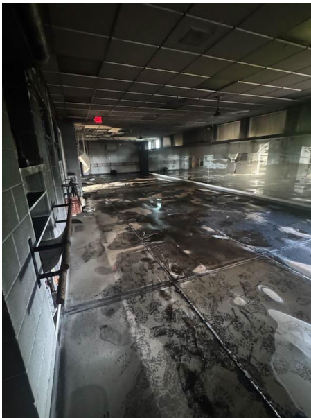
Photo: A long interior hallway with charred, soot-covered walls and a wet, stained floor from fire and water damage.
