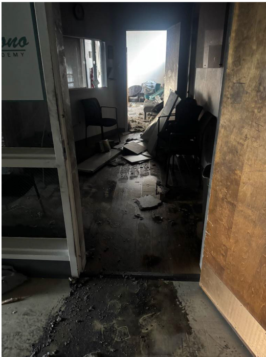
Photo: A fire-damaged office area viewed through a charred doorway, with debris and burned materials scattered on the floor.
