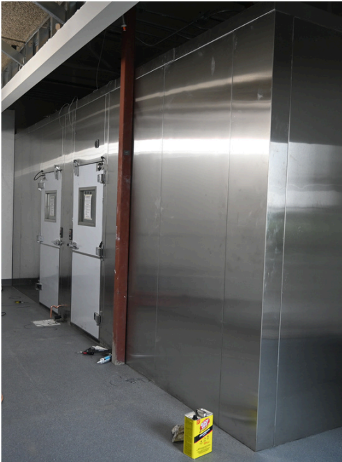
Walk-in cooler installed at Salnave Elementary as part of the kitchen expansion.
