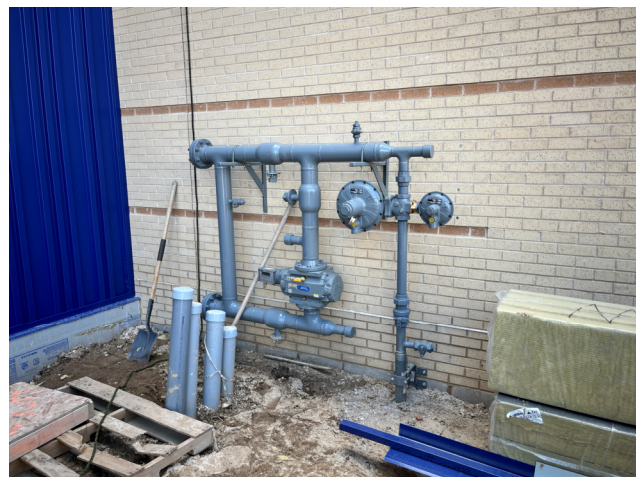
Gas Meter – East Elevation Of Area C2
