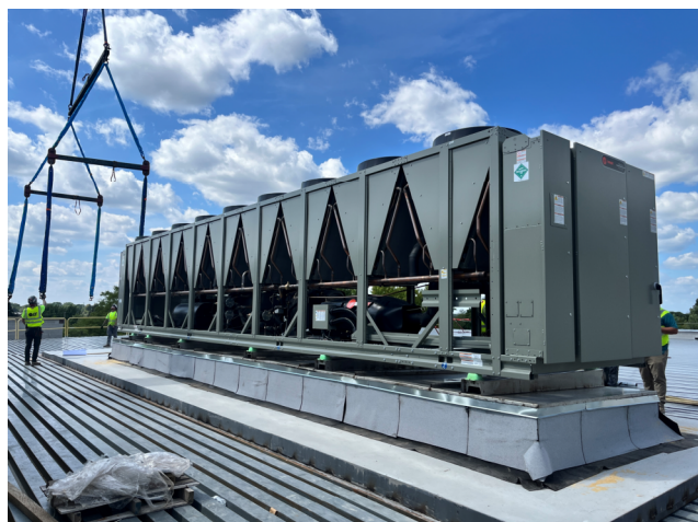
Chiller – Area C2 Roof
