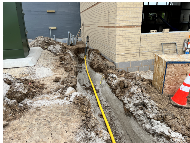
Main Gas Pipe – North Of Area A2
