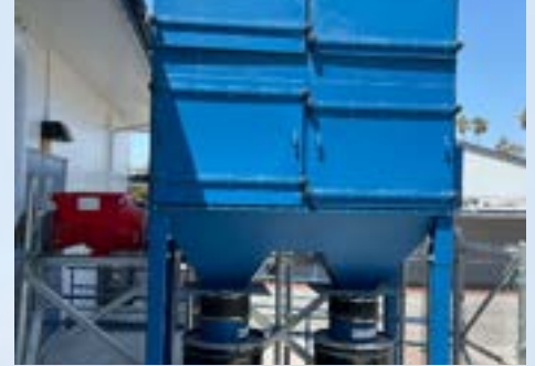
Adolfo Camarillo High School Dust Collection System
