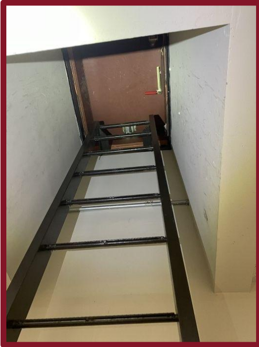
Roof Hatch Lock
