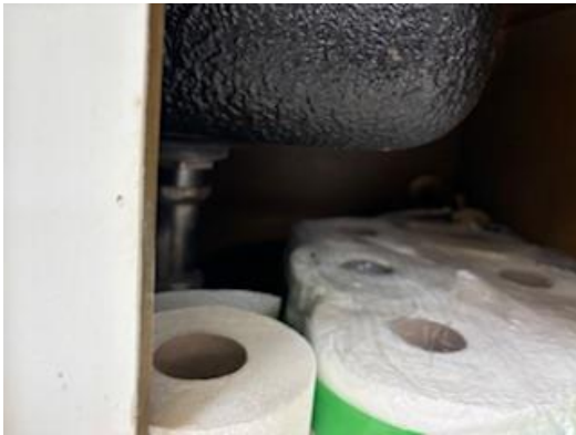
#13 View of HA-24: Asbestos-containing Black Sink undercoat (6% Chrysotile)
