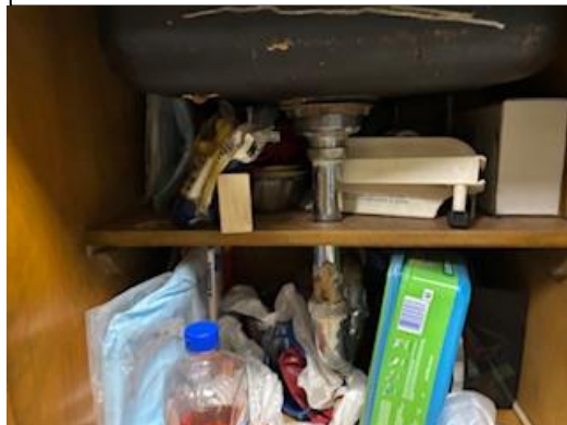
#11 View of HA-19: Brown Sink Undercoat
