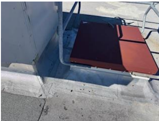
#27 View of PC-03 Red Paint on Metal Roof Hatch
