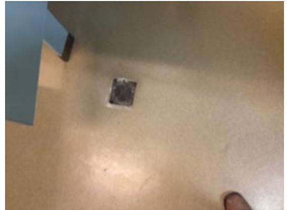
#20 View of HA-43 Epoxy Flooring
