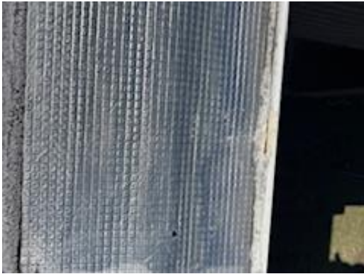
#1 View of HA-01: White Flashing Sealant
