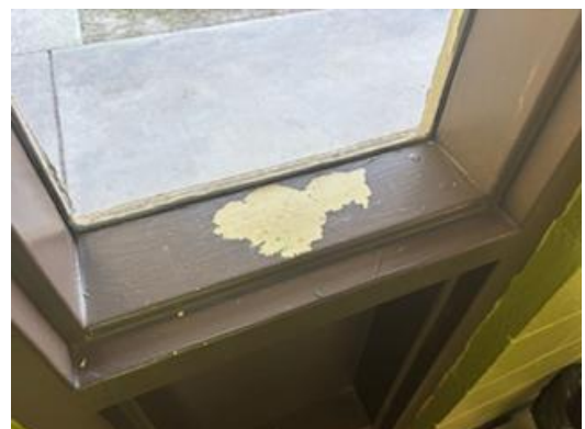
#30 View of PC-15 Brown Paint on Metal Window Frame
