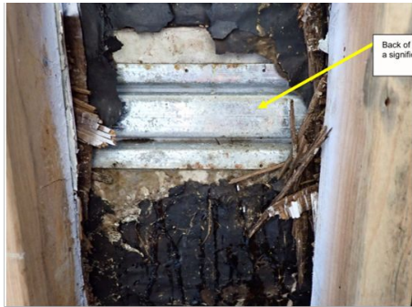
Rotted sheathing at stucco reveal; water flowed inside during testing.
