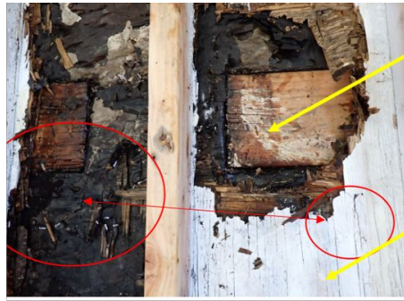
Water entered around wood blocking, nail penetrations and lag bolts.
