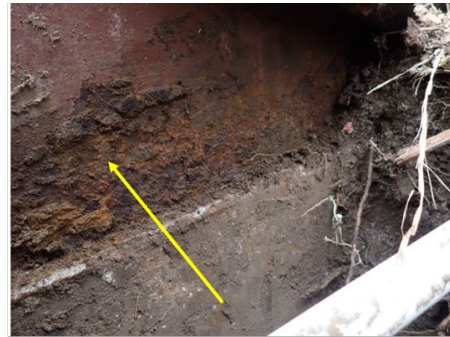
Corrosion of the steel C-channel; no waterproofing observed.
