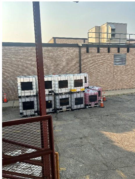
Chiller Glycol 100% Filled
