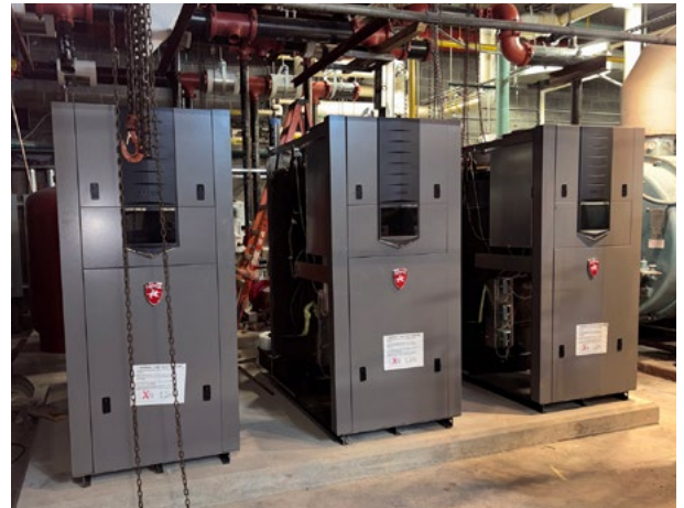
Amherst Middle steam-to-hot water conversion.
