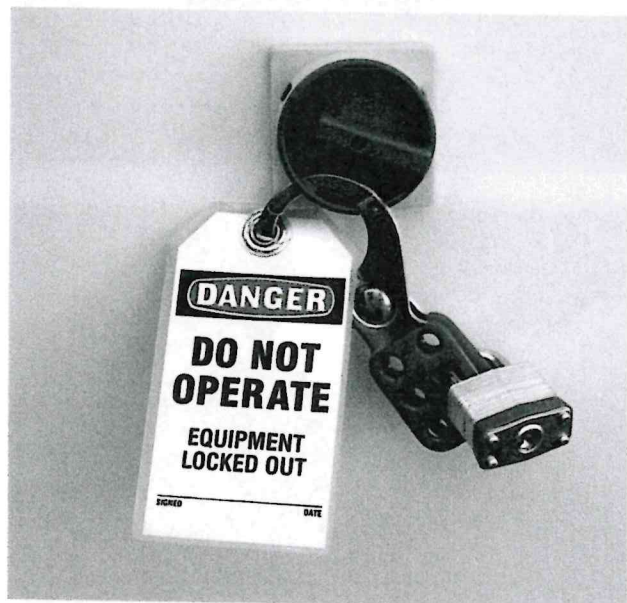
FIGURE 14-4 Some facilities use a lockout tag system for damaged equipment to prevent anyone from using the equipment.
