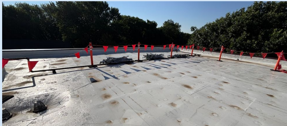
Woodlawn Solar Installation
