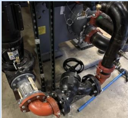
Lawrence High School Chillers
