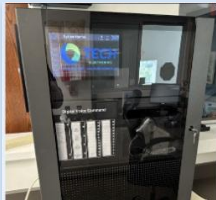
Cordley Fire Alarm System
