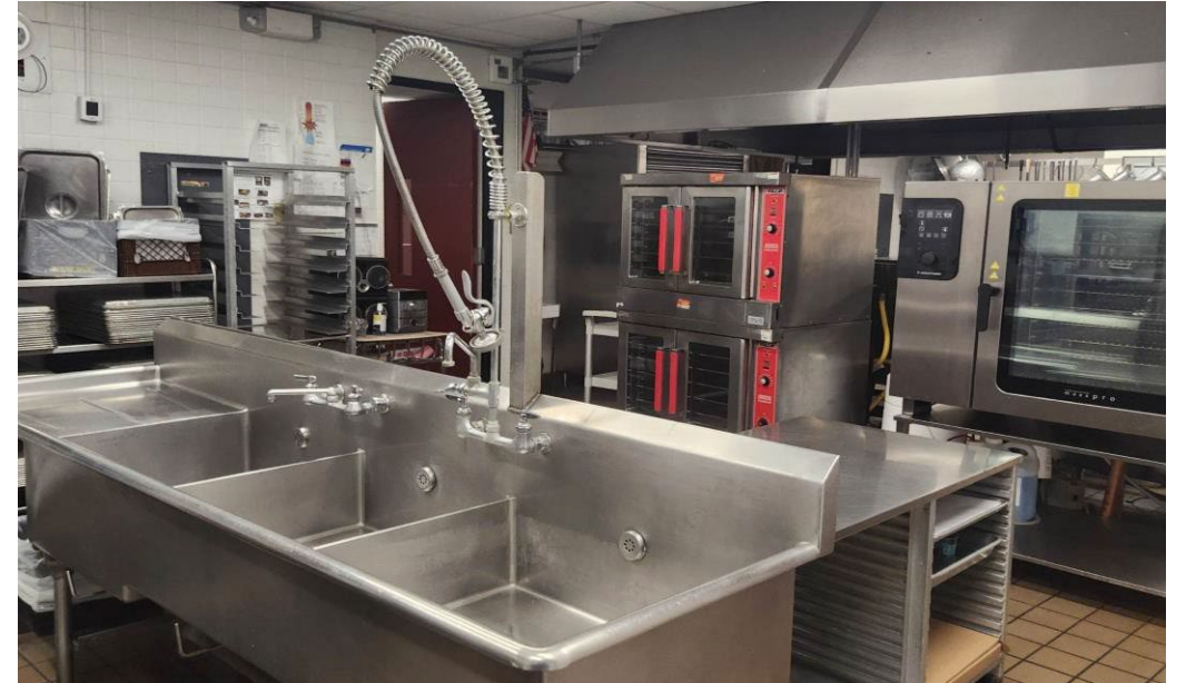
New Kitchen Equipment and Replace Hood (Existing Equipment shown here)
