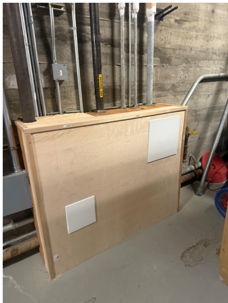
A sealed box was installed to limit air exchange between room and tunnel.
