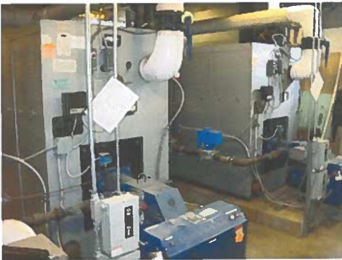
Heating water boilers
