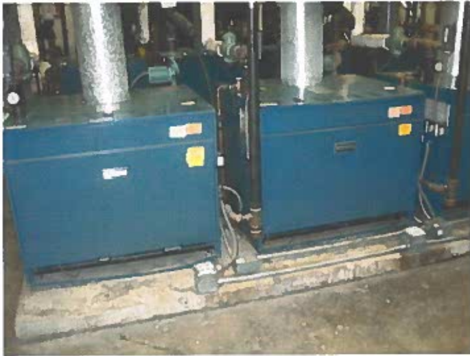
Heating Water Boilers
