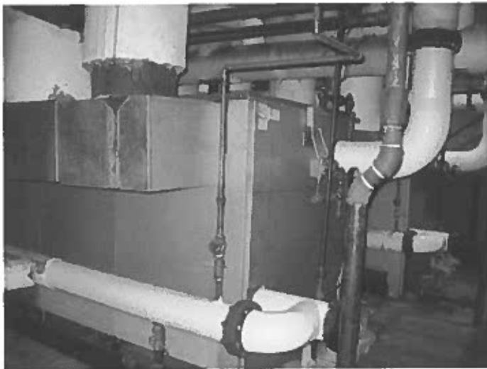
Steam heating boilers
