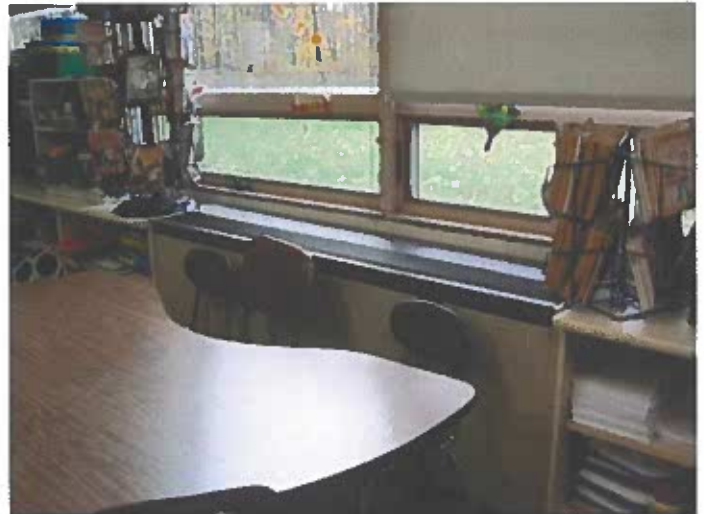
Classroom Univ Ventilator
