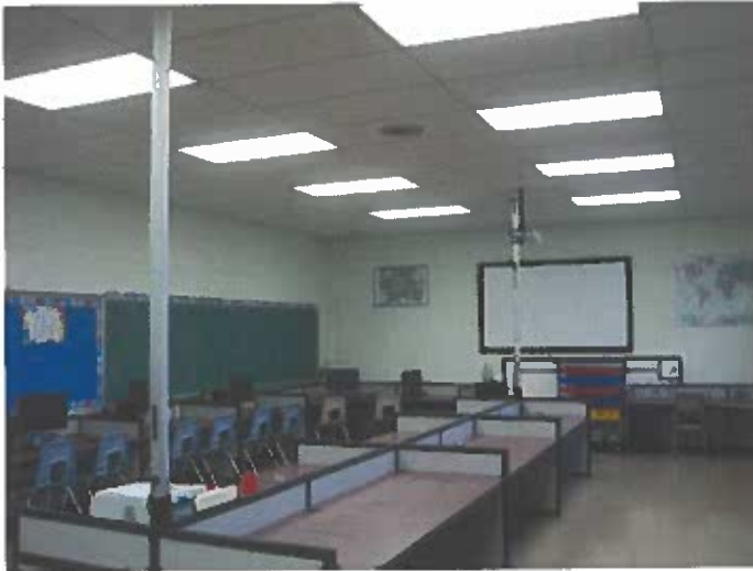
Typical CR lighting
