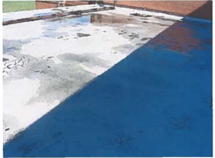
Standing Water on Adhered Membrane
