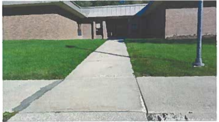
Typical Sidewalk Condition
