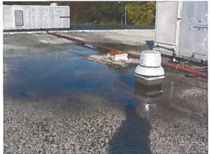
Standing Water on Ballasted Membrane
