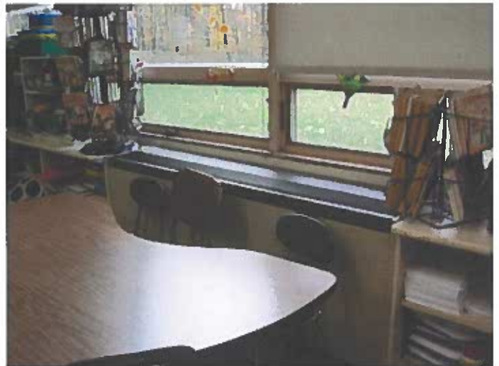
Classroom Univ Ventilator
