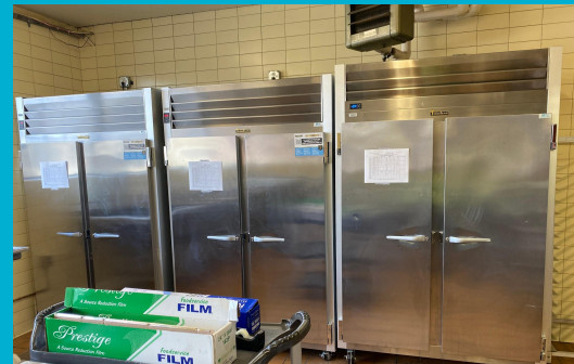
Reach-in freezer (3 units)
