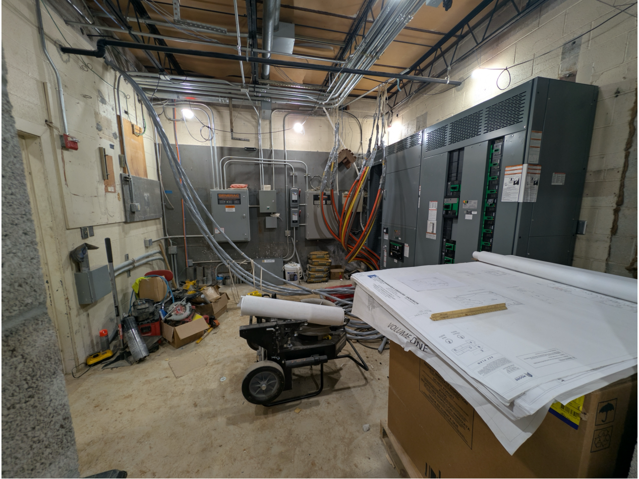
New Electric Equipment In New Electric Room
