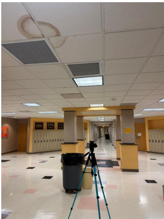
Hall near C106, active leak
