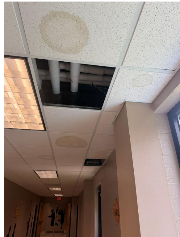
Stained ceiling tile in Hallway outside A102
