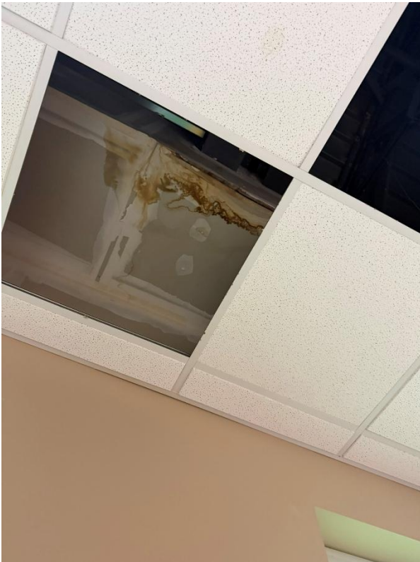
D117 Workroom – staining on sheetrock above ceiling tile with potential active leak
