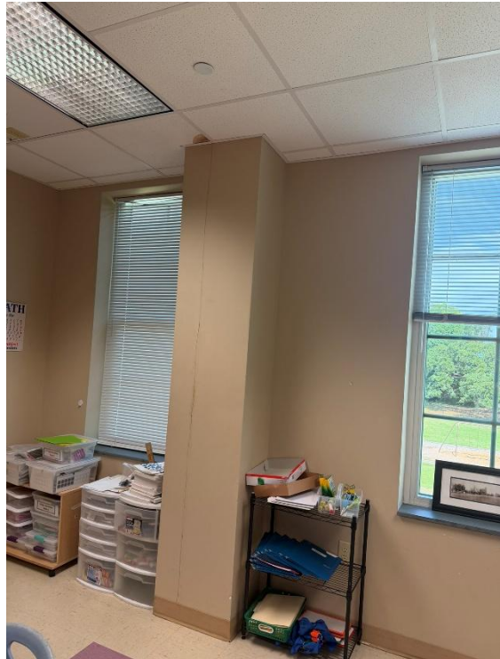
B214 – stained ceiling tiles and drip staining on wall
