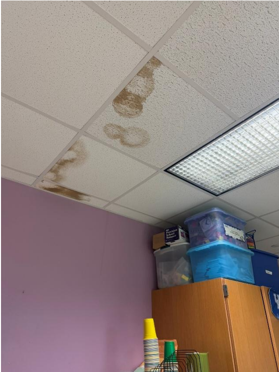
B214 – stained ceiling tiles
