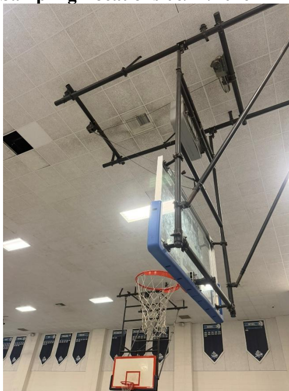
Gym – particulate at supply vents
