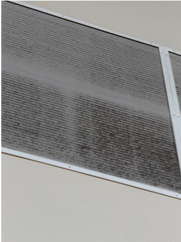
Gym – Particulate on grille
