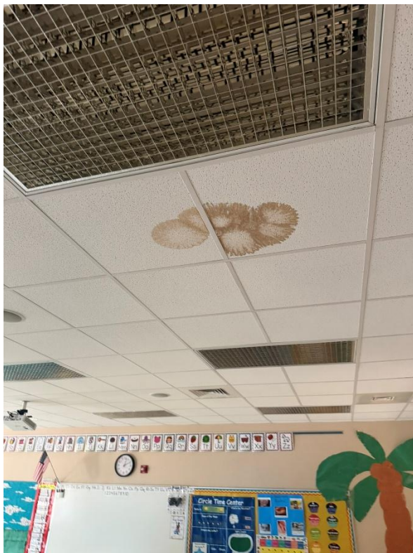
Classroom 133 – stained ceiling tiles
