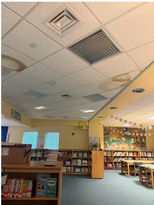
Media Center – stained ceiling tiles
