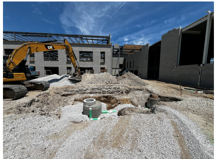
Storm Drain – Site – South Of Main Entrance
