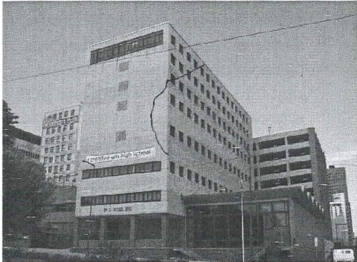
Structural damage to 65 Kellogg
