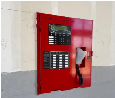
Fire Alarm Panel
