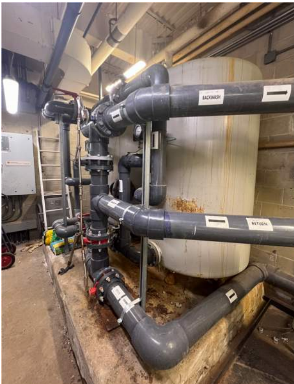
Photo 27: Pool water is filtered through two, dual-cell, high rate sand filters. Each cell has 12.57 sf of sand bed for a total of 50.28 sf. At a flow rate of 635 GPM, the filter operates at 12.63 GMP/sf, which is an acceptable filtration rate.
