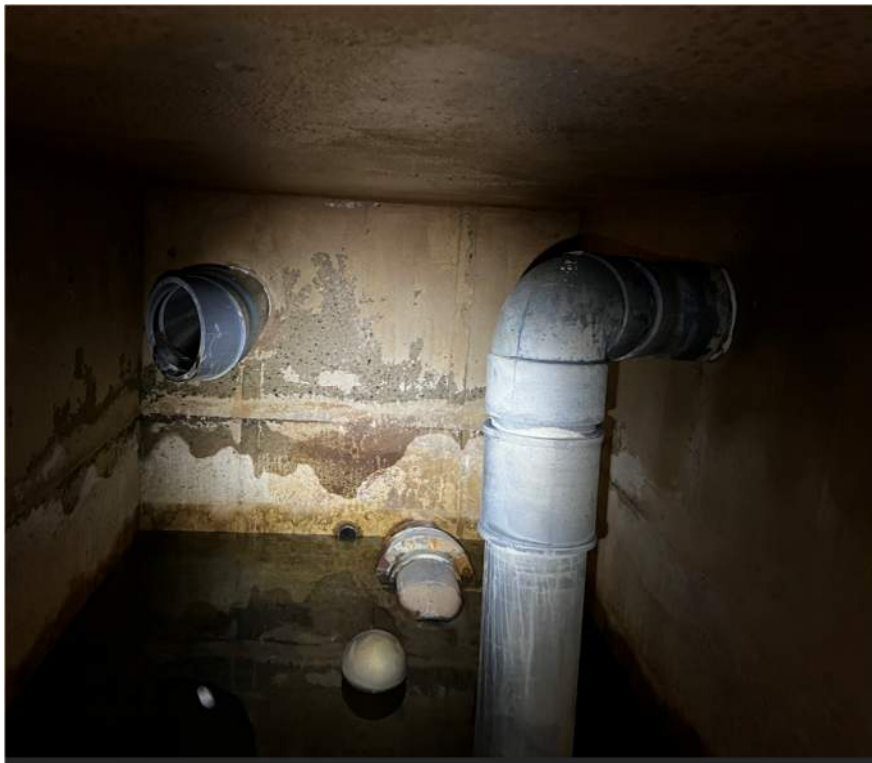
Photo 25: The surge tank is comprised of two, pre-cast concrete tanks with manhole access at grade. The two tanks communicate by means of connection pipes that allow water to equalize in the tanks. Water gravity flows from the gutter drains into the tank. Main drain flow enters the tank through a modulating valve.
