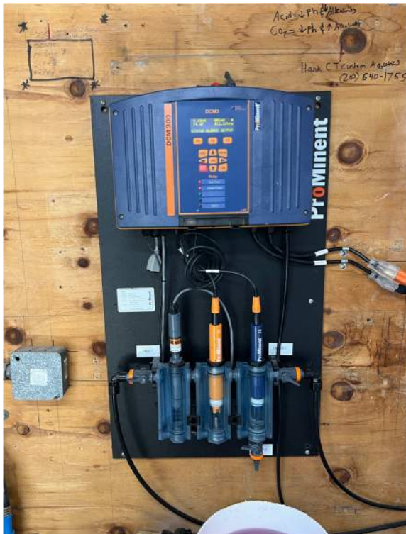
Photo 31: Chemicals are automatically monitored and fed through a chemical controller. The Prominent Unit installed at the pool is relatively new and is appropriate for continued use.
