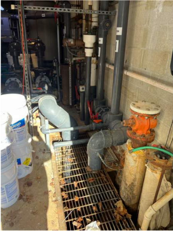
Photo 24: (Left) Pipe pit provides an area way for piping into and out of surge tank, which is located below grade south of the Filter Room Wall.
