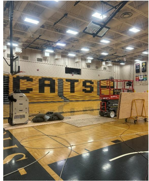
Ductwork Clean HS Gymnasium
