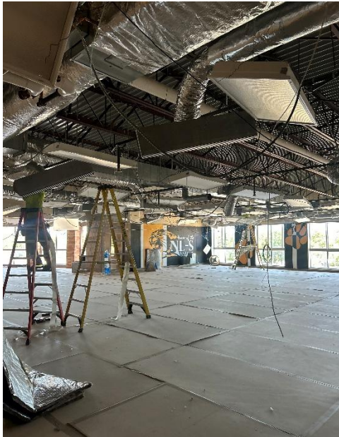
Ductwork Insulation in Cafeteria
