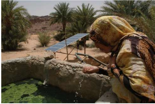
FIGURE 65.5 Solar panels in Africa. In areas where the electrical grid is not established and electricity supply lines are not present, the installation and use of photovoltaic solar cells may be less expensive and less environmentally disruptive than a traditional electrical infrastructure. (Pallava Bagla/Corbis)
