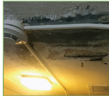
Roof leaks in the Carmel High School music building.
