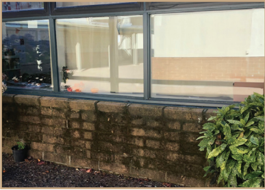
Deteriorating adobe walls and single pane windows at Carmel High School
