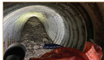
Aging storm drains at Captain Cooper starting to collapse
