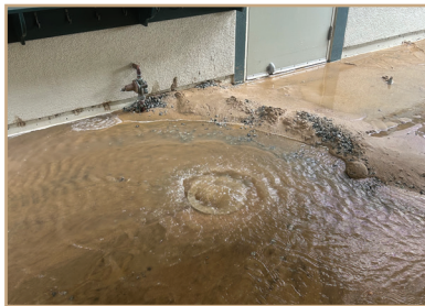
Aging pipes caused flooding in the walk area and some classrooms at Carmel River Elementary School
