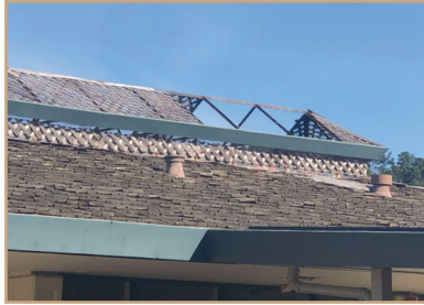
Damaged cupola on Carmel Middle School roof
