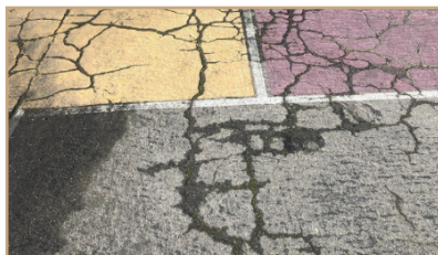
Asphalt walkway trip hazards at Tularcitos Elementary
