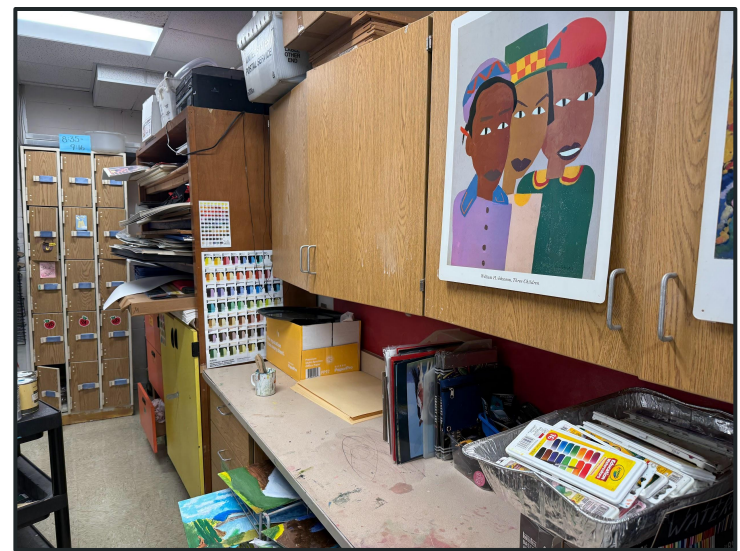
Existing Middle School Art Classroom ceiling condition.
