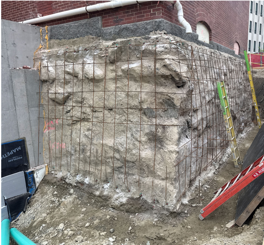
May 14: Wear Wall at SW Corner of Historic Building
