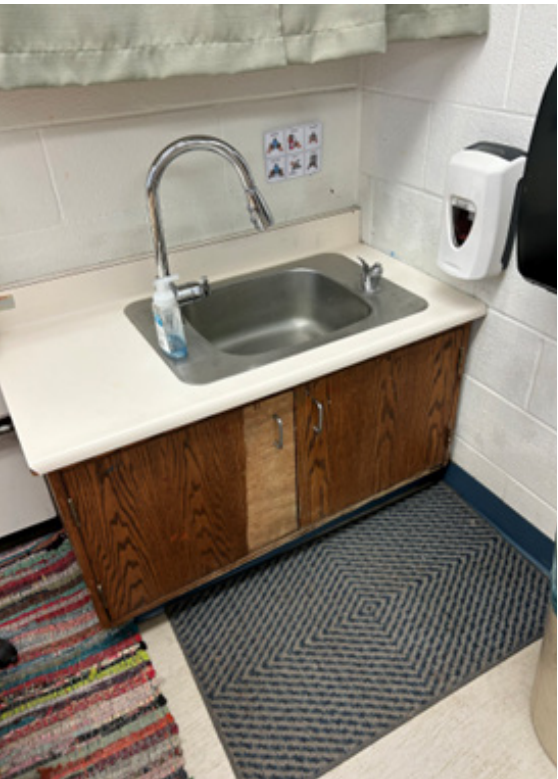
Built-in cabinets are original, delaminating, damaged and limited, which minimizes the ability to store classroom materials.
