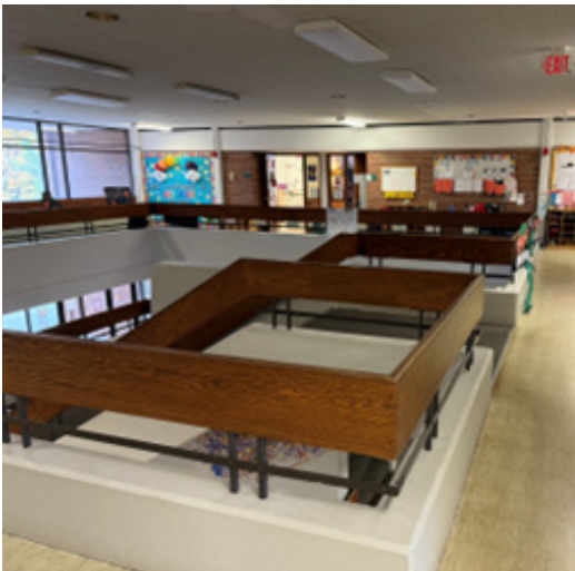
Guardrail height below Building Code
