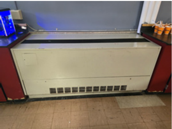
Inefficient unit ventilators need replacement
