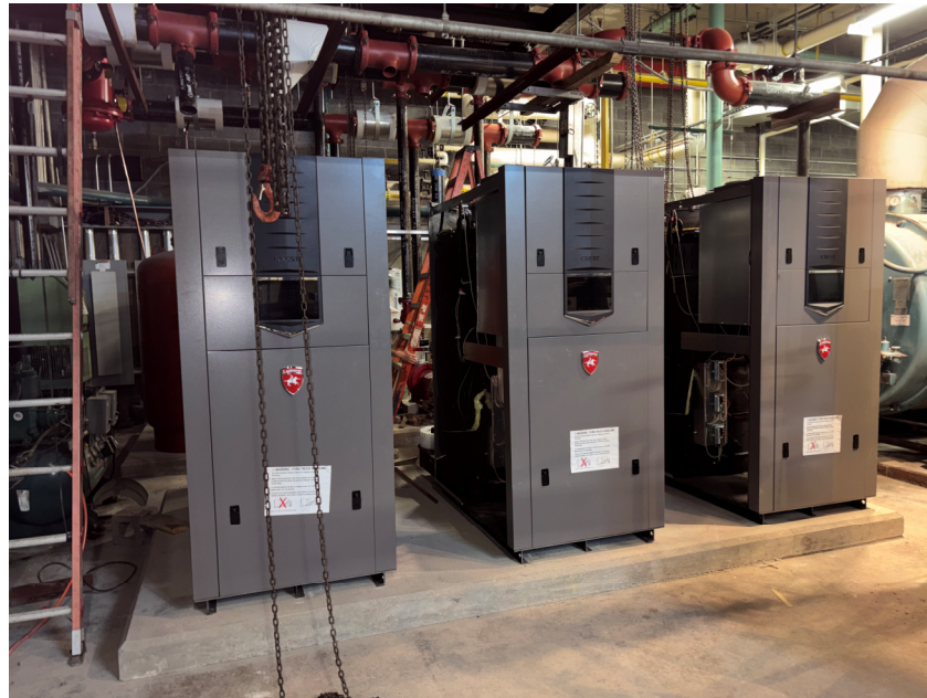
MS New HW Boilers
