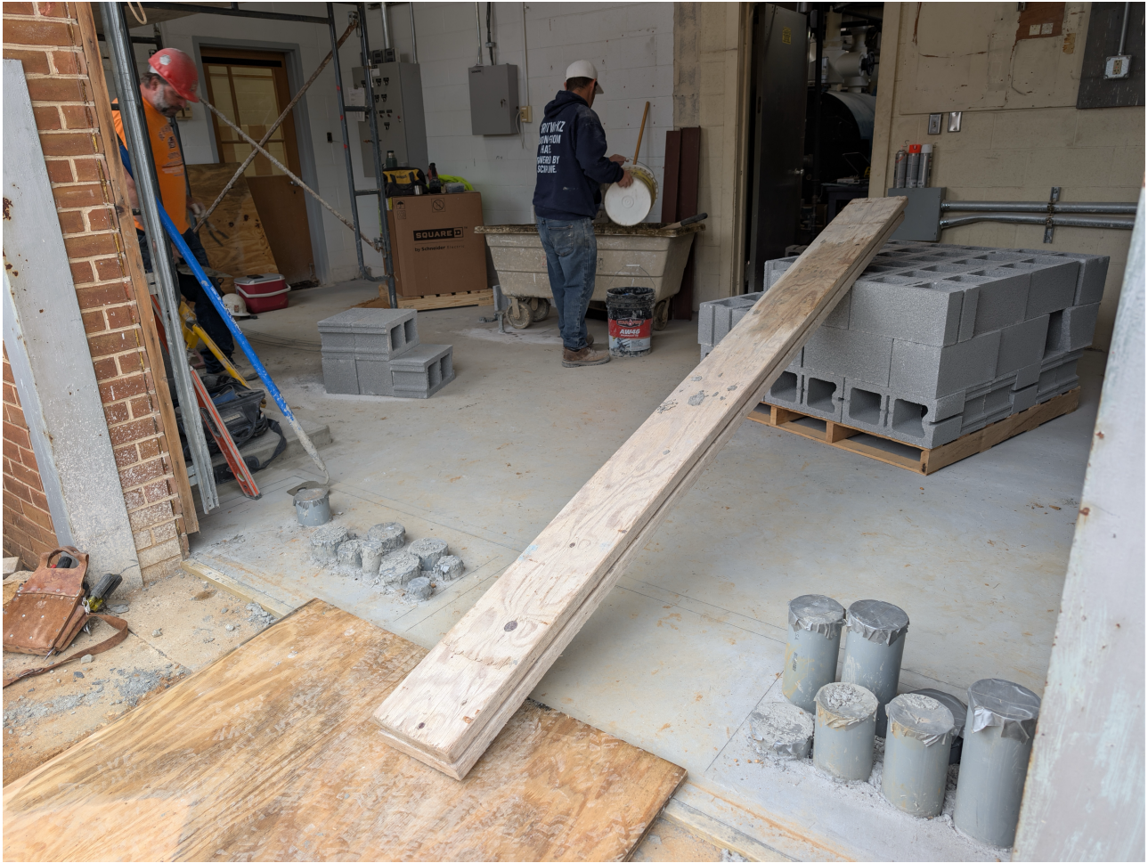
New Electric Room in Existing Building
