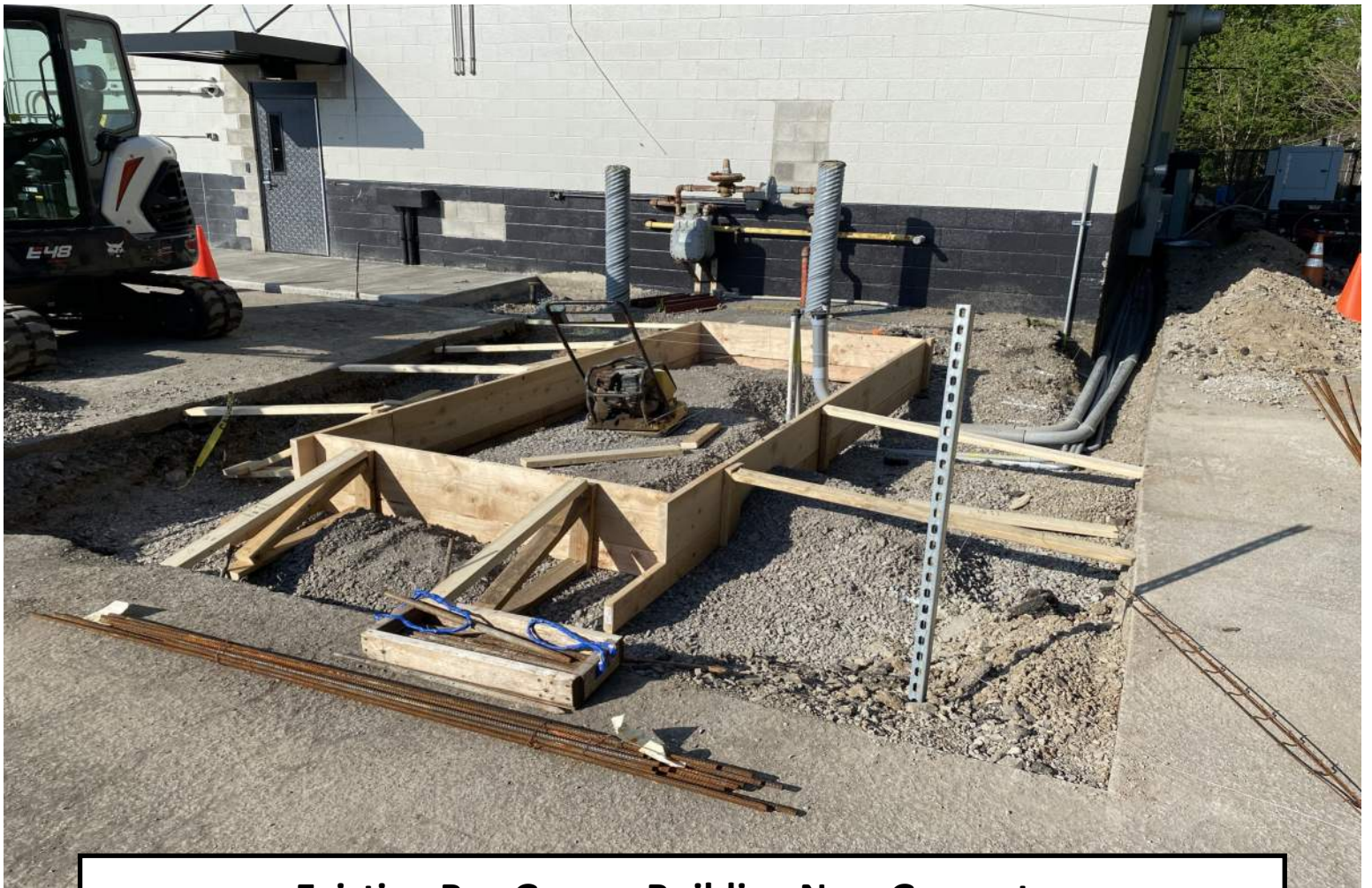
Existing Bus Garage Building New Generator
