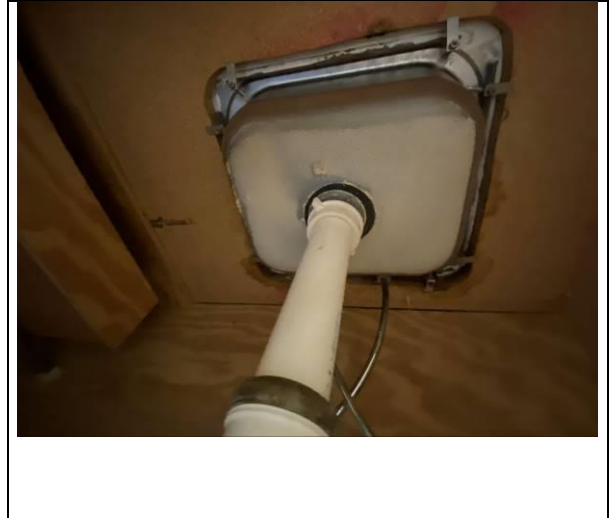
Photo #8. View of assumed ACBM white under sink coating on sink in the office area.
