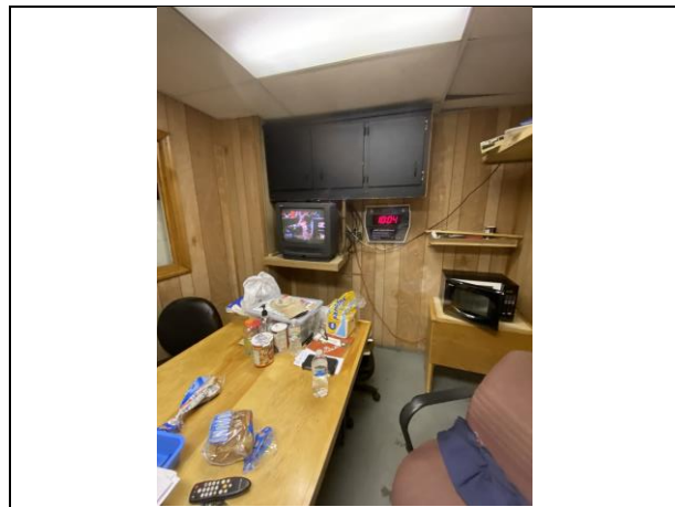
Photo #18. View of assumed ACBM observed in the Shop breakroom.
