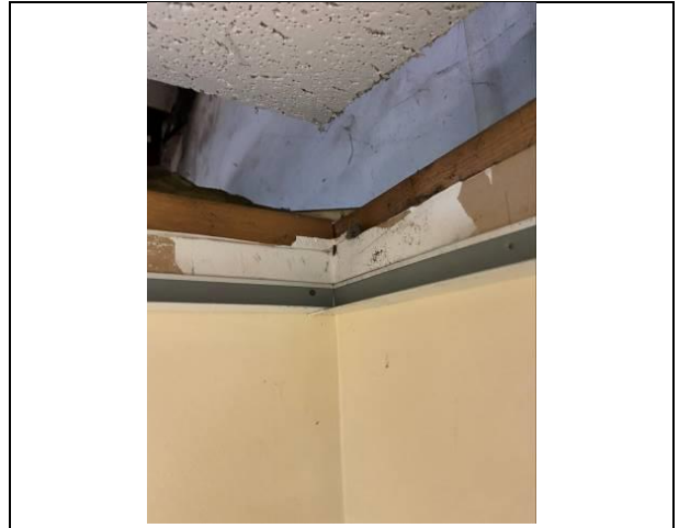
Photo #4. Typical assumed ACBM yellow/tan sheetrock and white joint compound.
