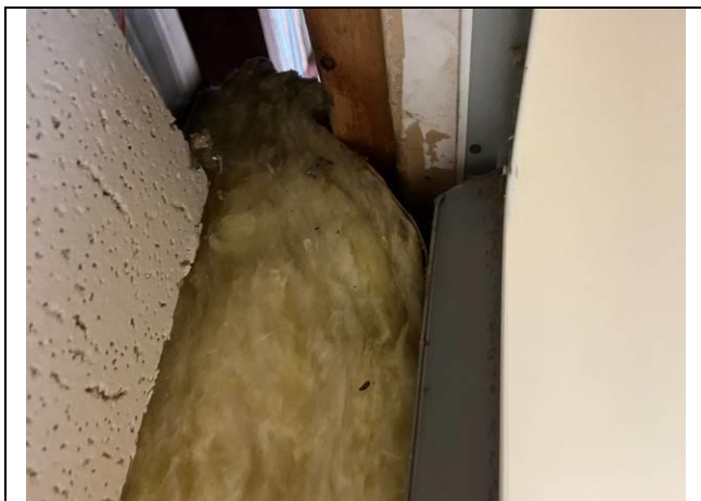
Photo #5. Typical assumed yellow insulation above ceiling tile in the office area.
