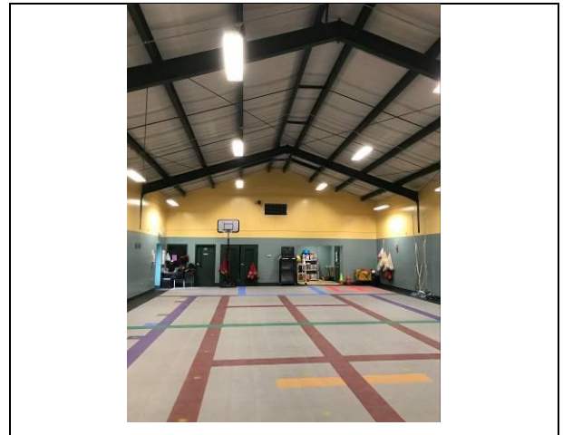
Photo #4. View of assumed ACBM within the gym.
