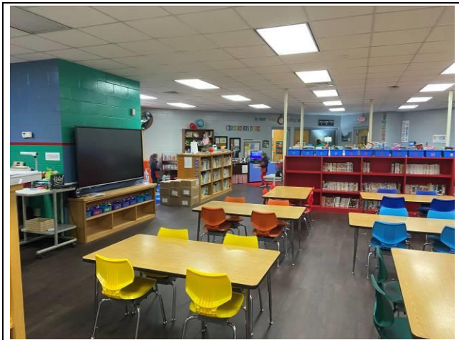
Photo #9. View of assumed ACBM dark brown laminate in the Media Center, room 300.
