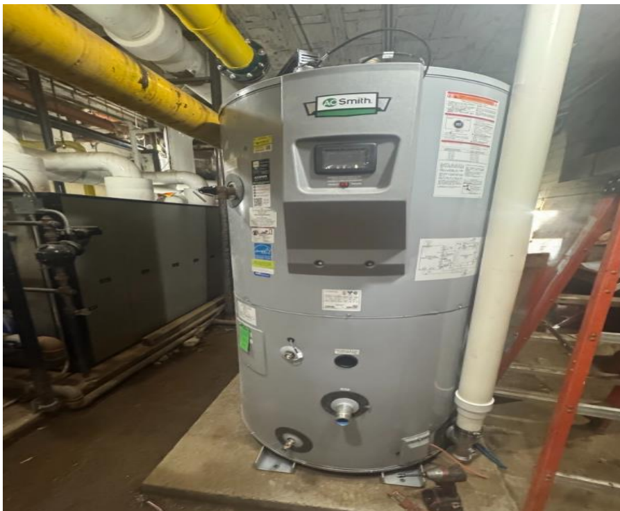
Hempstead ABGS MS – Boiler Room Equipment
