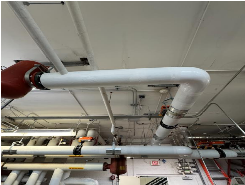
Hempstead IAQ – Chilled water piping
