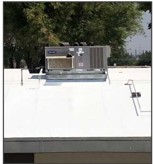
New HVAC Units
