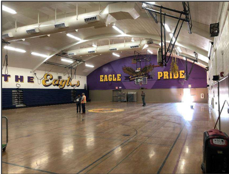
Existing Gym with new HVAC
