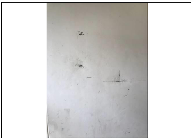
Photo #5. Positive plaster on exterior of media center with minor damage.
