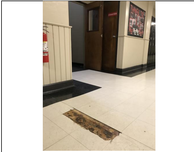
Photo #13. View of typical damaged assumed ACBM vinyl tile found throughout the school.
