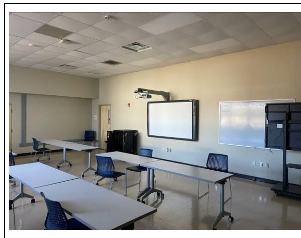
Photo #10. View of assumed sheetrock and joint compound in added wall room 314.
