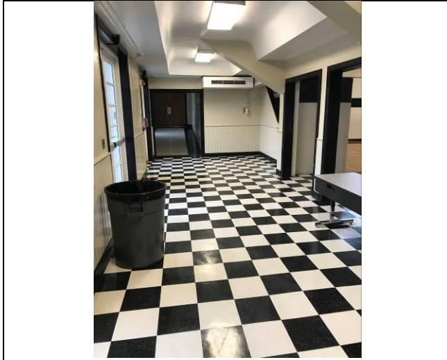
Photo #7. View of assumed ACBM vinyl floor tile in old gym lobby.
