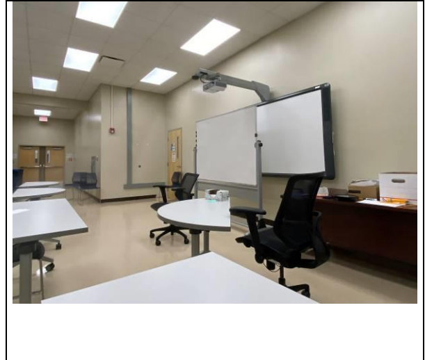
Photo #8. View of assumed tan painted white sheetrock/ joint compound in room 312 added wall.
