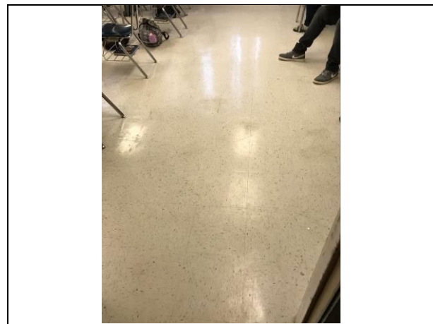
Photo #12. View of assumed ACBM vinyl floor tile in room A106 in history hall.
