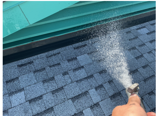
Water tested louver and counter flashing - leak did not activate
