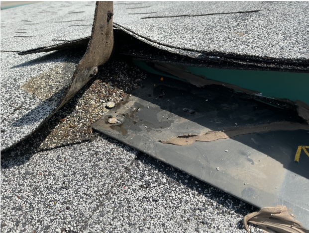
Removed first piece of hip, revealing that the area is wide open for water to enter the roof system
