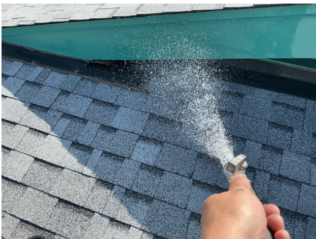
Water tested corner of louver and soffit - leak did not activate
