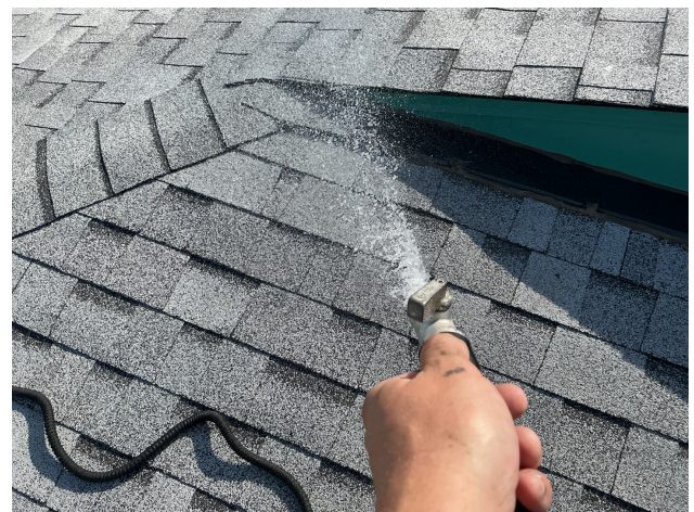
Water tested corner of hip cap where it meets the green metal - leak immediately activated inside cafeteria
