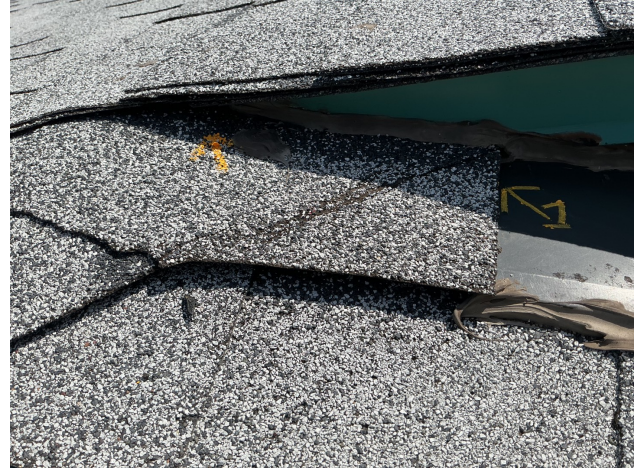
Corner of louver flashing was allowing water to enter the roof system
