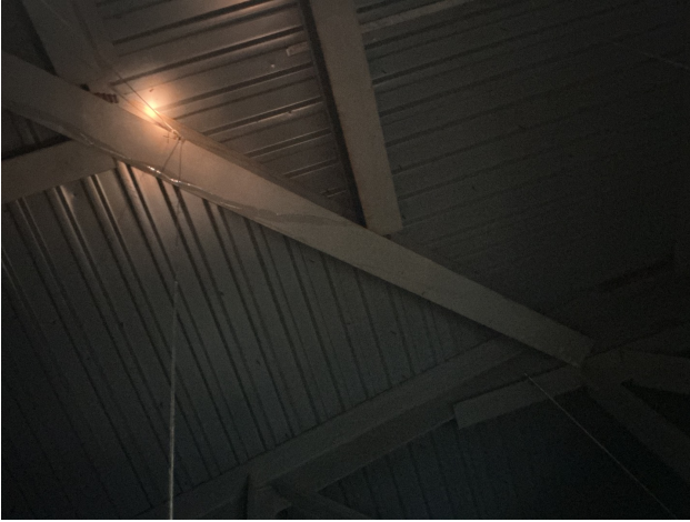
Water test performed and leaked an exact spot running down I-beam
