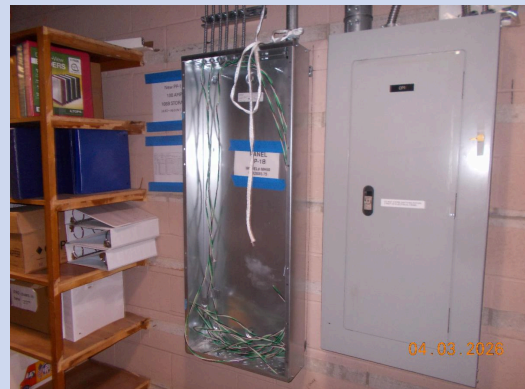
A new electrical panel at Brunner.
