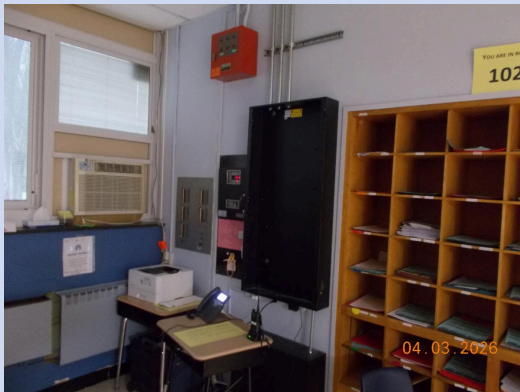
New fire alarm control panel at Coles.
