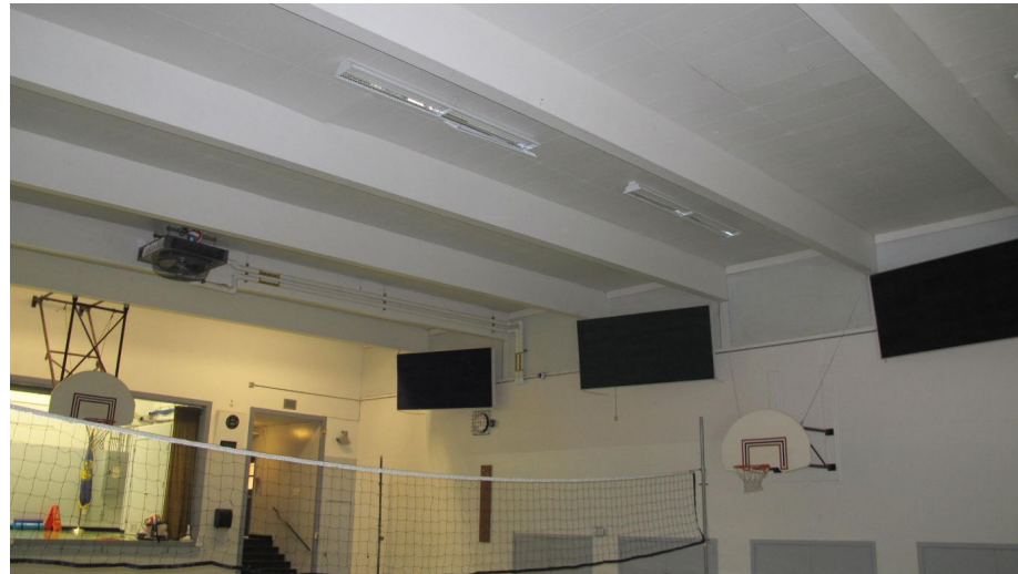
Reference Photo 1 - Brattain Campus / Gateways High School: mechanical piping conditions that may interfere with end brackets. Drawings have been revised to allow for fasteners to be moved to avoid the conflict, see revised 1/S8.01.
