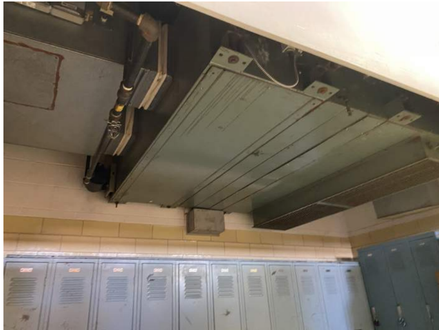
● D2. 3: Air Handling Unit Serving a Locker Room in Poor Condition.
