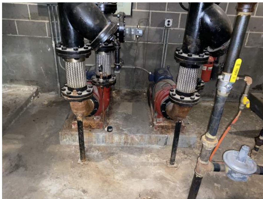
● D2. 36: Hot Water Pumps in Poor Condition.
