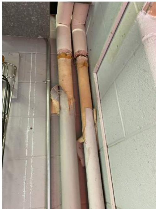
● D2. 35: Hot Water Piping in Poor Condition.
