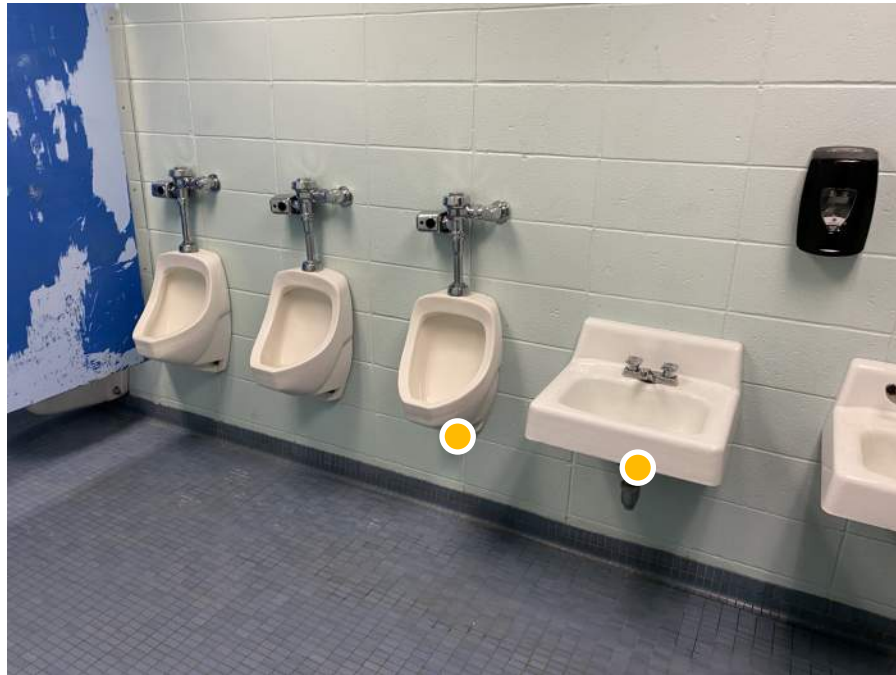
● D2. 51: Detail view of fixture replacement retrofit, does not meet all current accessibility codes.
