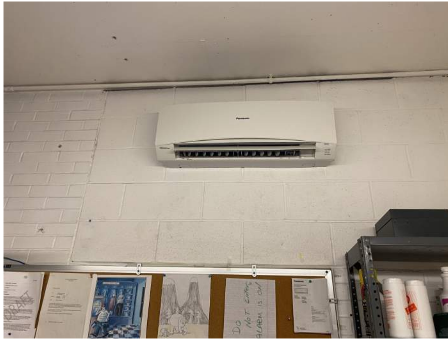
● D2. 67: Wall Mounted Split Unit For Cooling in IDF Room.
