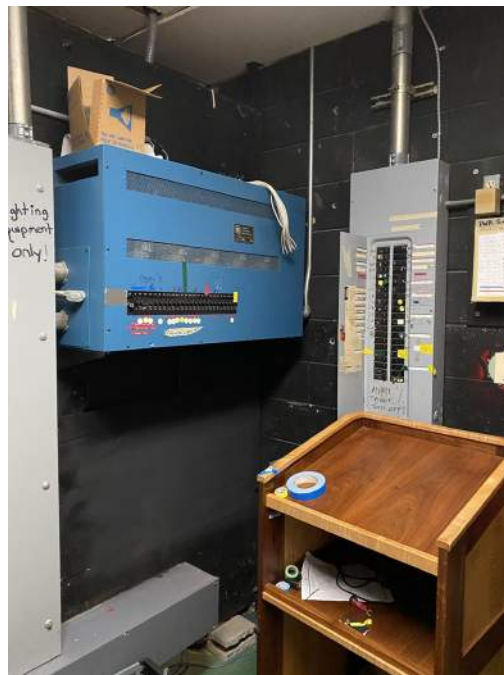
● D2. 18: Electrical Stage Power and Control.
