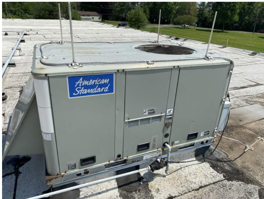
● D2. 4: American Standard Rooftop Unit in Poor Condition.
