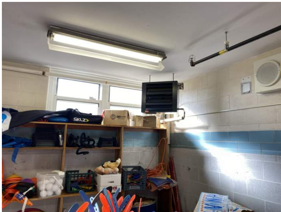
● D2. 38: Hot Water Unit Heater in Fair Condition.
