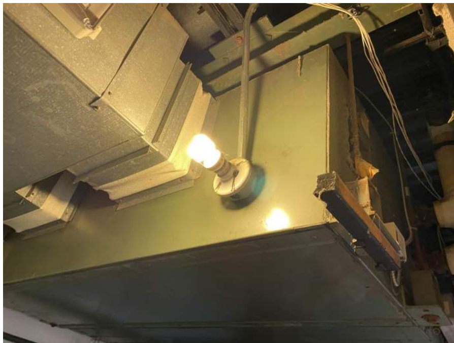
● D2. 2: Air Handling Unit Serving Girls Locker Room in Poor Condition.
