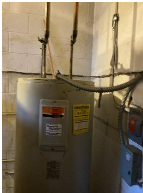
● D2. 8: Domestic Water Heater in Poor Condition.
