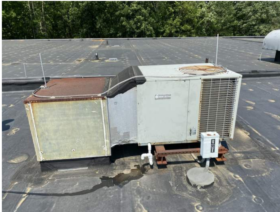
● D2. 57: Small Trane Unit in Poor Condition.
