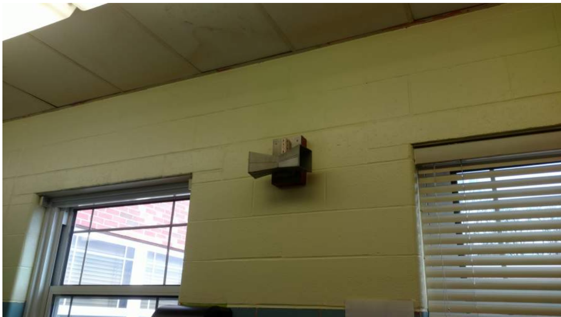
● D2. 50: Old School Fire Alarm.
