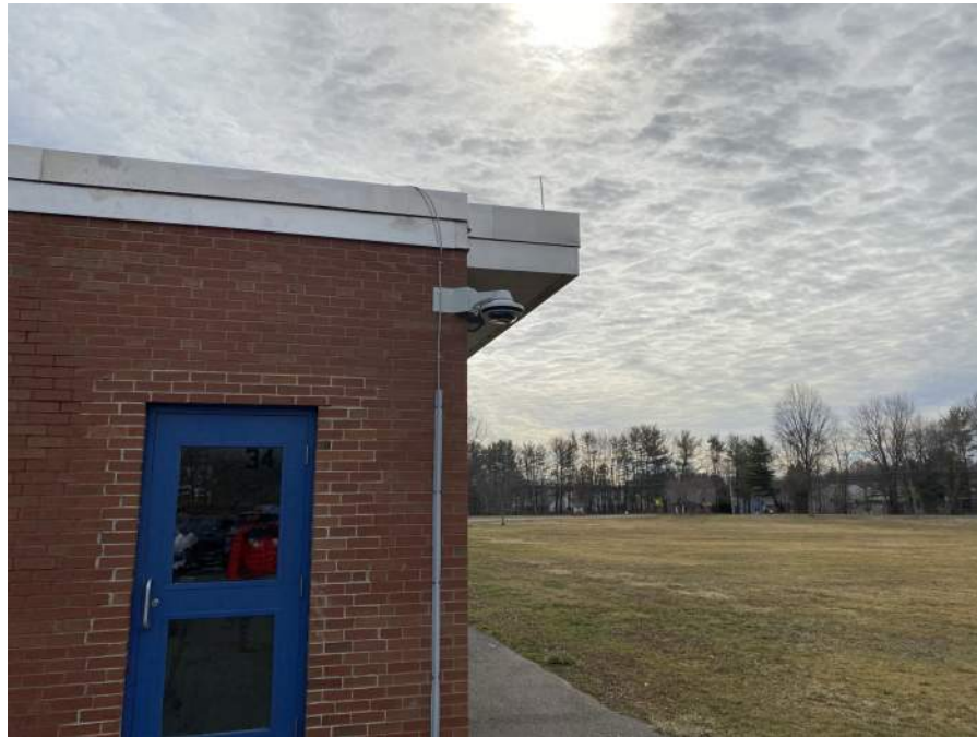
● D2. 23: Exterior Security Camera.
