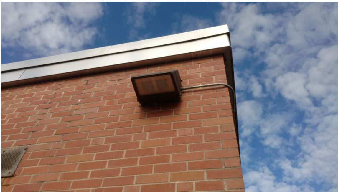
● D2. 22: Exterior LED Wallpack Lighting.
