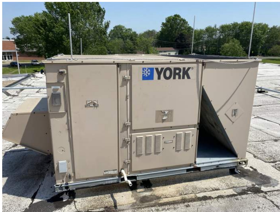
● D2. 64: Typical York Rooftop Unit in Poor Condition.
