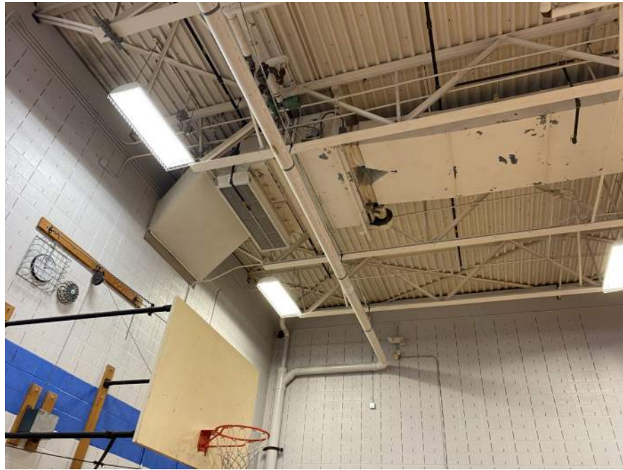
● D2. 27: Gymnasium Air Handler and Ductwork in Poor Condition.
