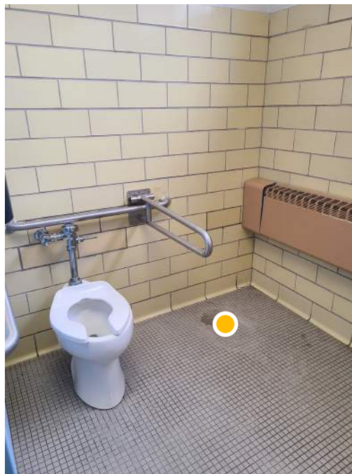
● D1. 60: Detail view of toilet fixture reconfiguration to meet accessibility codes, note floor patching and repairs
