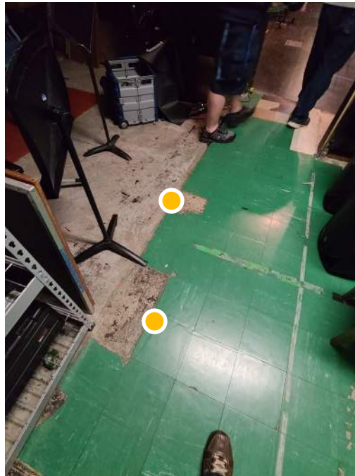
● D1. 61: Detail view of IT storage and server room with VAT flooring retrofits.
