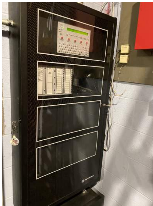
● D2. 24: Fire Alarm Control Panel.
