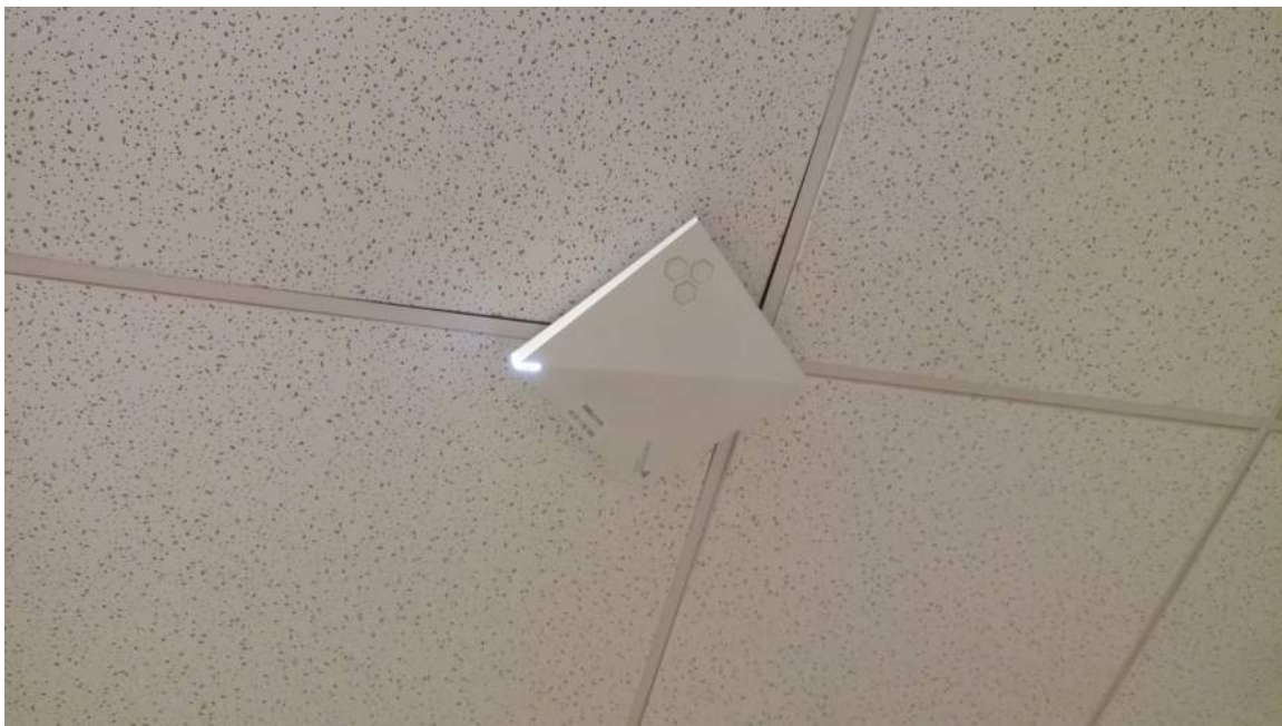
● D2. 68: Wireless Access Point.
