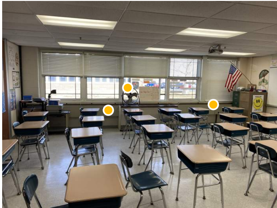
● D2. 63: View of typical classroom with unit ventilator and perimeter radiation units at exterior wall, note the fan to compensate for additional air circulation.
