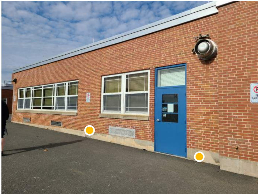
● D1. 5: View of typical exterior wall in 1965 Vo-ag addition. Note spalling concrete foundation wall
