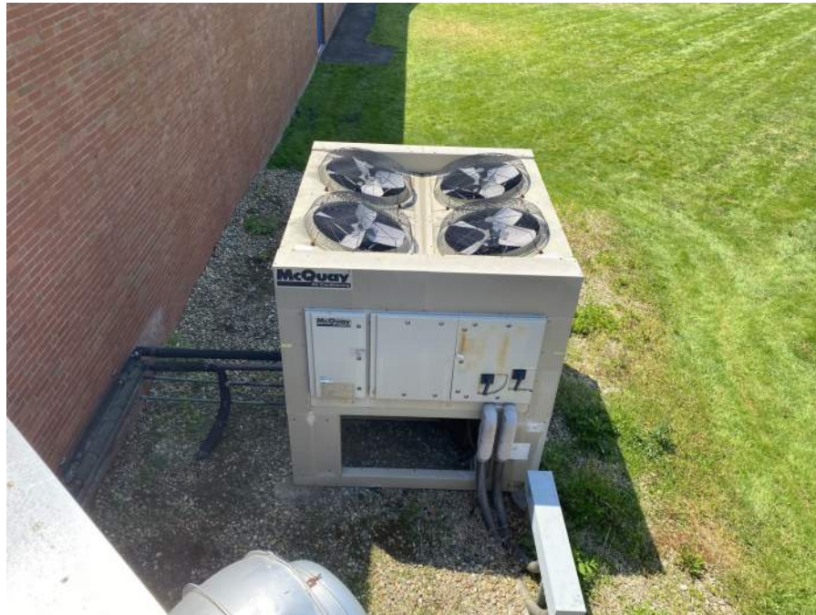
● D2. 47: McQuay Condensing Unit in Poor Condition.
