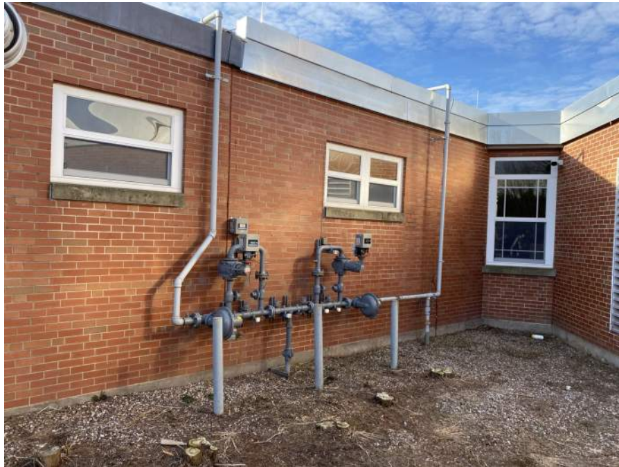
● D2. 49: Natural Gas Service.
