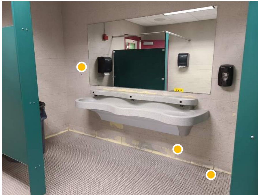
D1. 53: Typical bathroom retrofit in original two story classroom portion of the building, note the condition of the walls and floors
