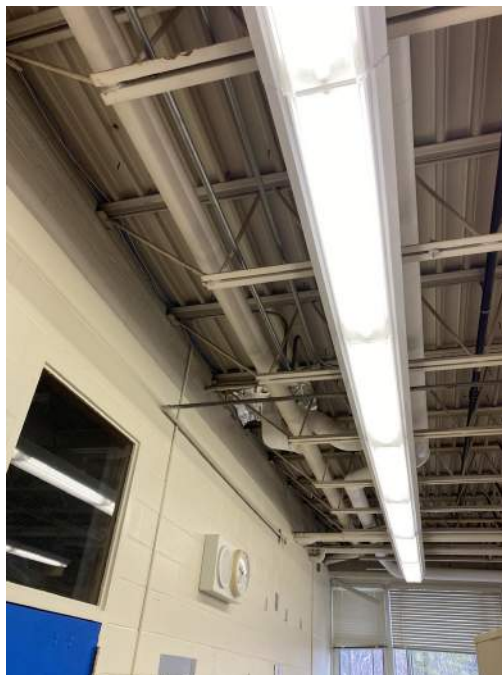
● D2. 58: Storm Piping from Roof Drain in Fair Condition.
