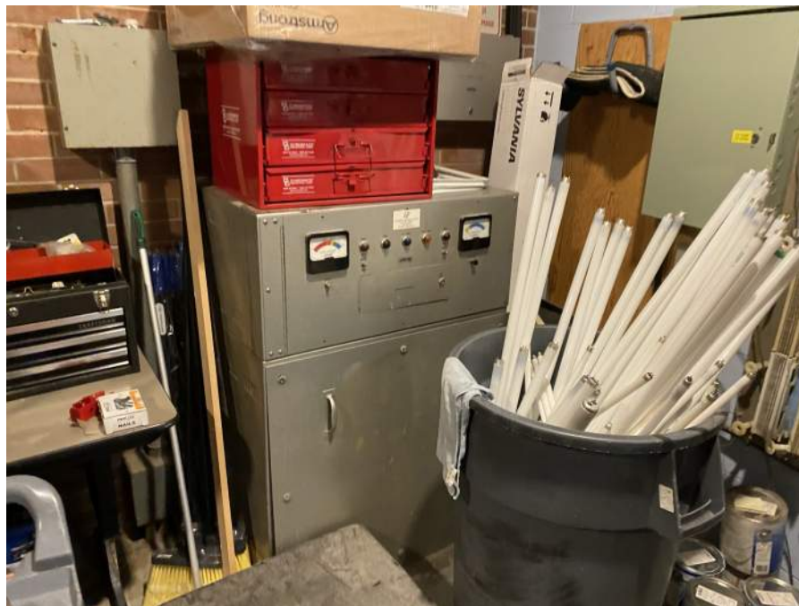
● D2. 20: Emergency Lighting Inverter System #1.
