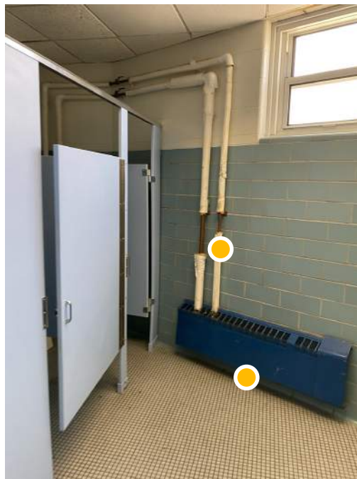
● D2. 32: Boys toilet room with exposed heating pipes to unit cabinet heater, adjacent to gymnasium, original construction 1964.
