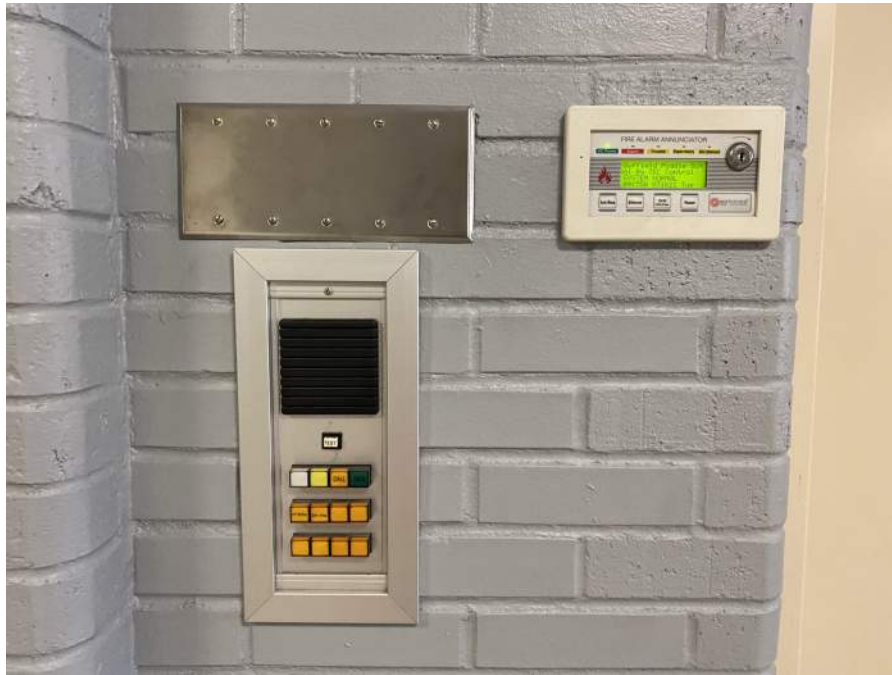
● D2. 5: Area of Rescue Assistance Intercom.
