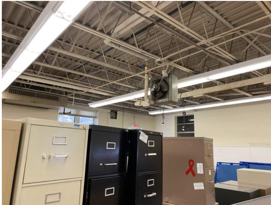
● D2. 37: Hot Water Unit Heater and Piping in Poor Condition.
