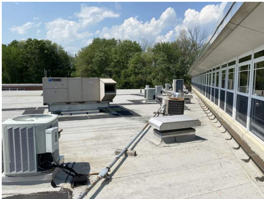
● D2. 66: Various Mechanical Equipment on Roof in Poor Working Condition.
