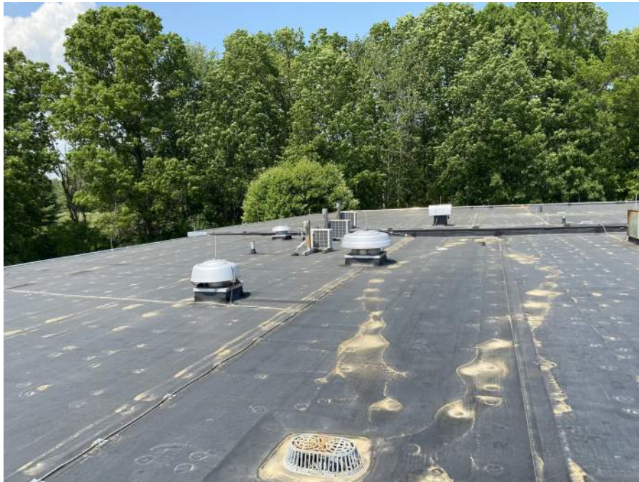
● D2. 21: Exhaust Fans and Condensing Units on Roof.
