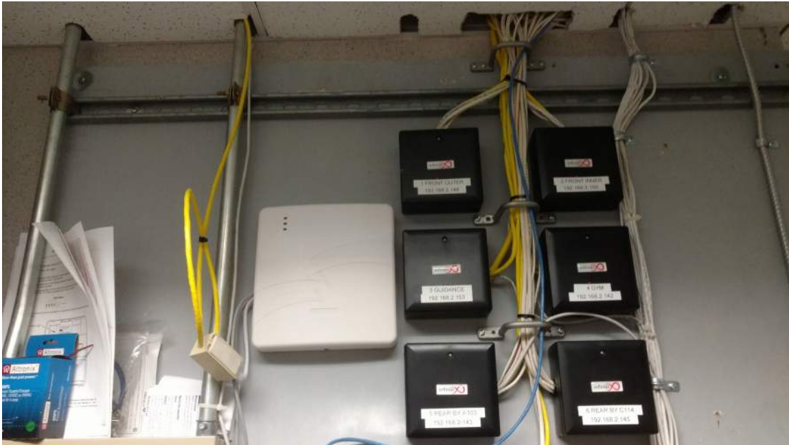
● D2. 1: Access Control Equipment.
