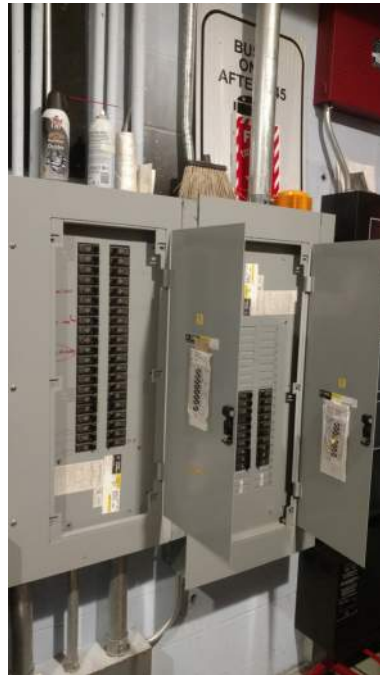
● D2. 13: Electrical Branch Circuit Panels.
