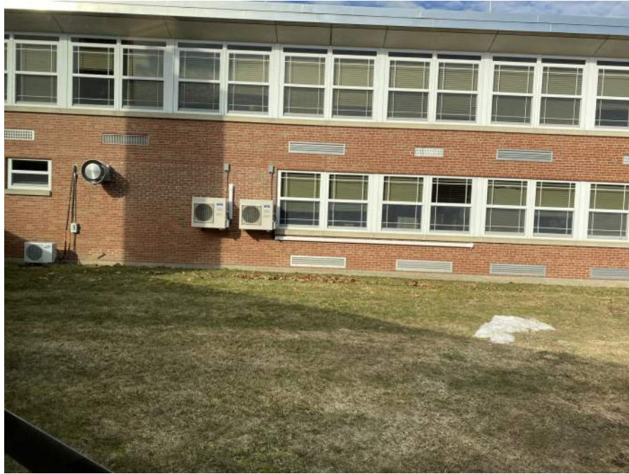
● D2. 65: Unit Ventilator and PTAC Unit Outdoor Air Intakes Along Wall.
