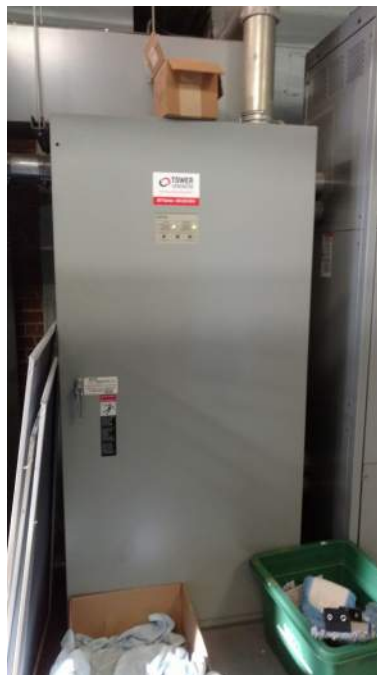
● D2. 12: Electrical Automatic Transfer Switch.
