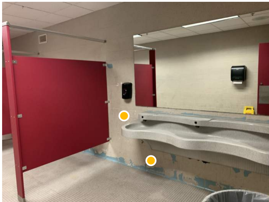
● D1. 68: Typical bathroom retrofit in original building of the building, note the condition of the walls.
