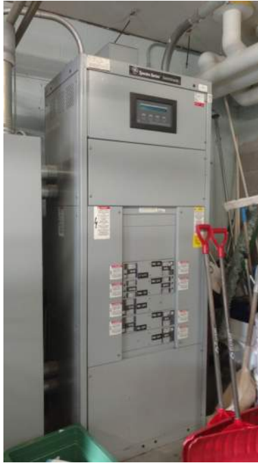
● D2. 19: Electrical Standby Power Distribution Panel.
