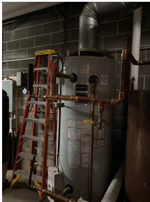
● D2. 48: Natural Gas Domestic Hot Water Tank in Mechanical Room.
