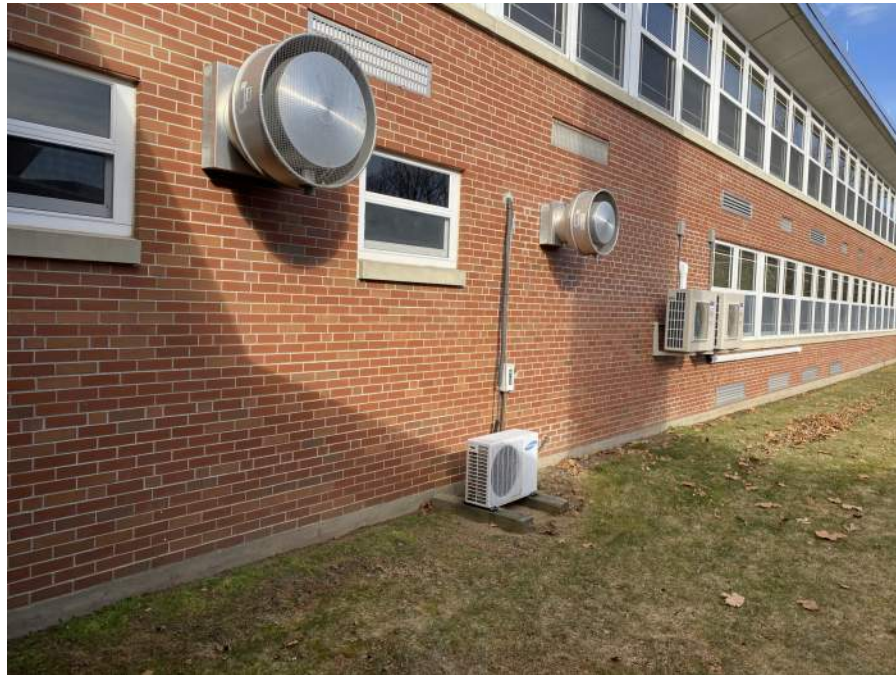
● D2. 7: Condensing Units and Wall Mounted Exhaust Fans Outside in Fair Condition.
