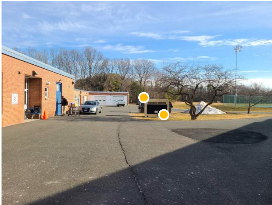
D3. 1: View of dumpster area along with generator, note no protection around ground mounted generator.
