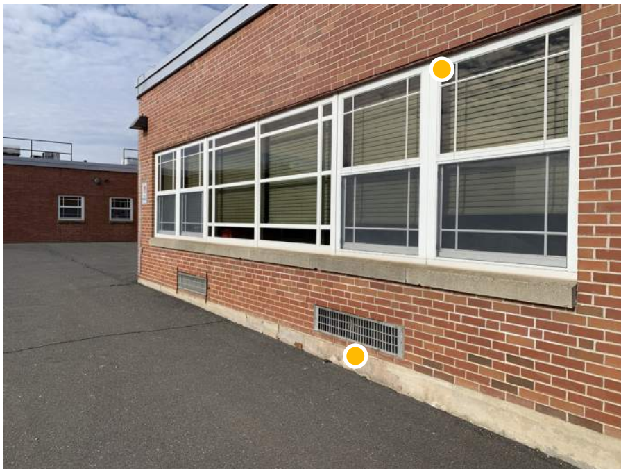
● D1. 6: Detail view of 1965 Vo-ag addition, note deteriorating steel lintels above windows and spalling concrete foundation wall below.
