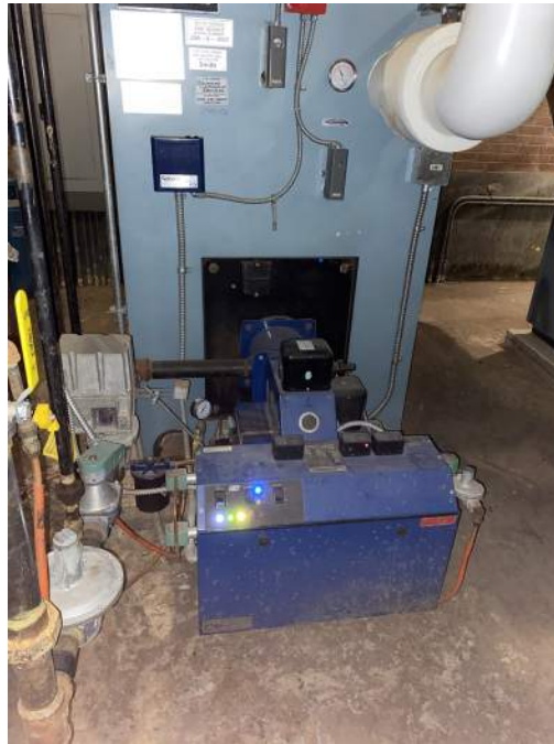
● D2. 31: Hot Water Boiler and Burner in Mechanical Room.
