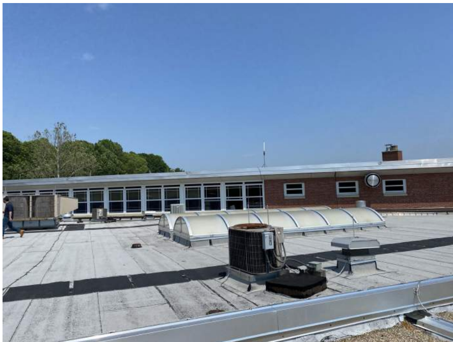
● D2. 54: Roof Mounted Condensing Unit in Poor Condition.
