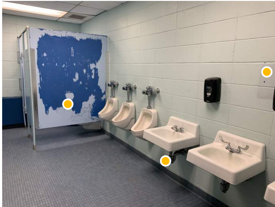
● D1. 67: Typical bathroom retrofit in original building, note the condition of the metal toilet partitions, does not meet current accessibility codes.
