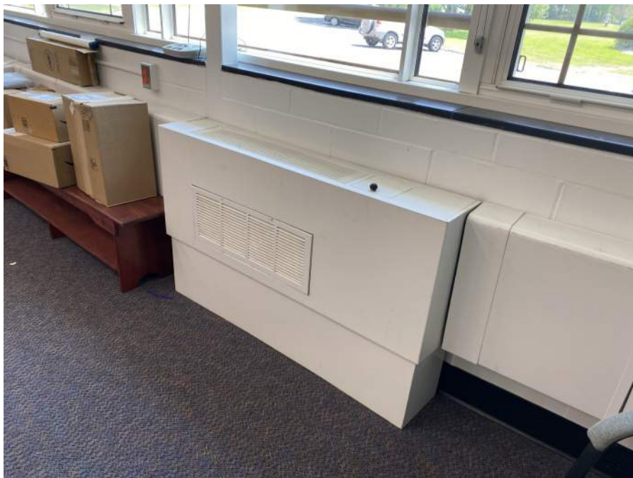
● D2. 62: Typical PTAC Unit in Poor Condition.
