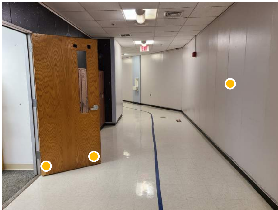
D1. 58: View of 1972 connecting corridor with modular wall construction, note condition of door and hardware.
