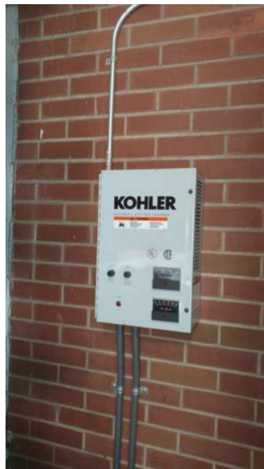
● D2. 14: Electrical Generator Remote Battery Charger.
