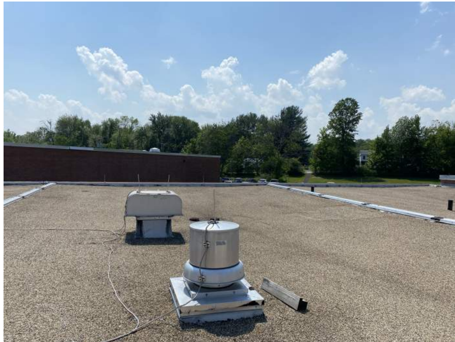
● D2. 55: Roof Mounted Exhaust Fans in Poor Condition.
