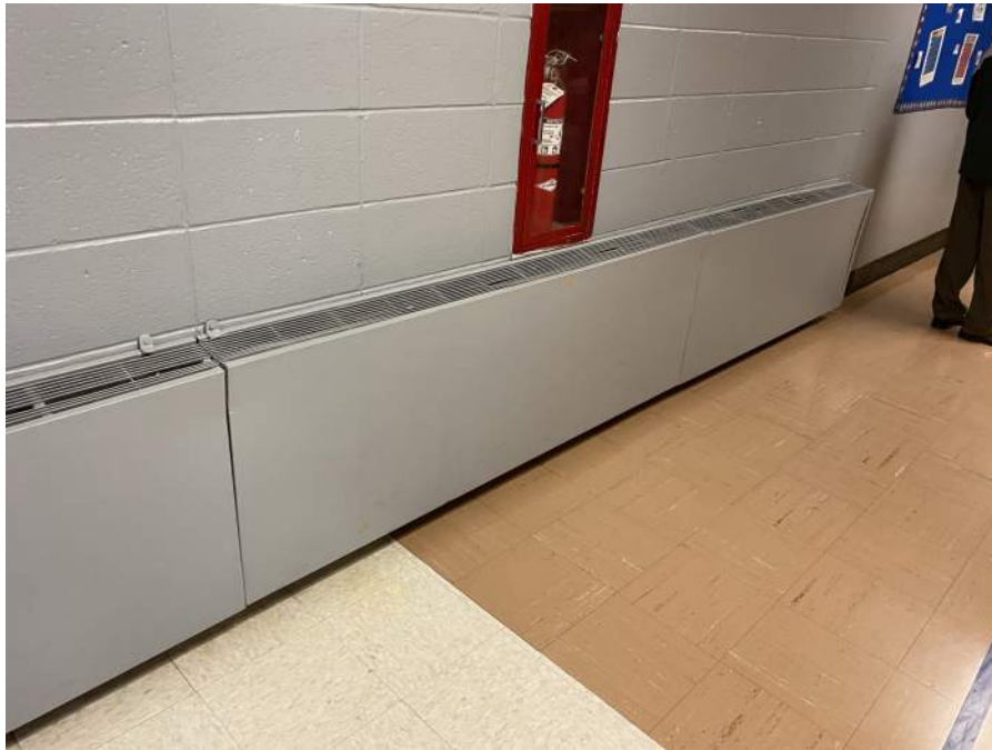
● D2. 33: Hot Water Convactor in Poor Condition.
