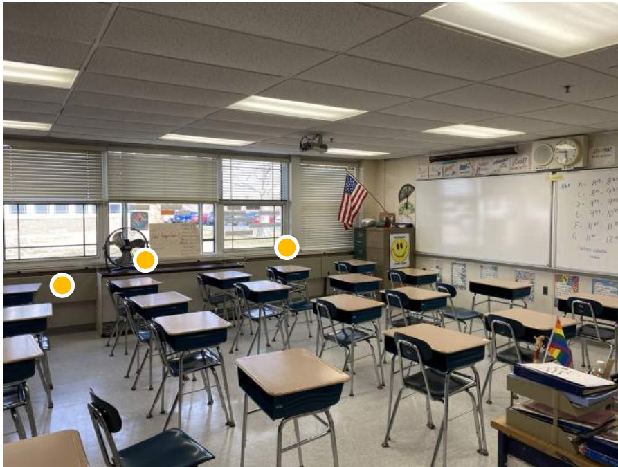
● D2. 61: View of typical classroom with unit ventilator and perimeter radiation units at exterior wall.
