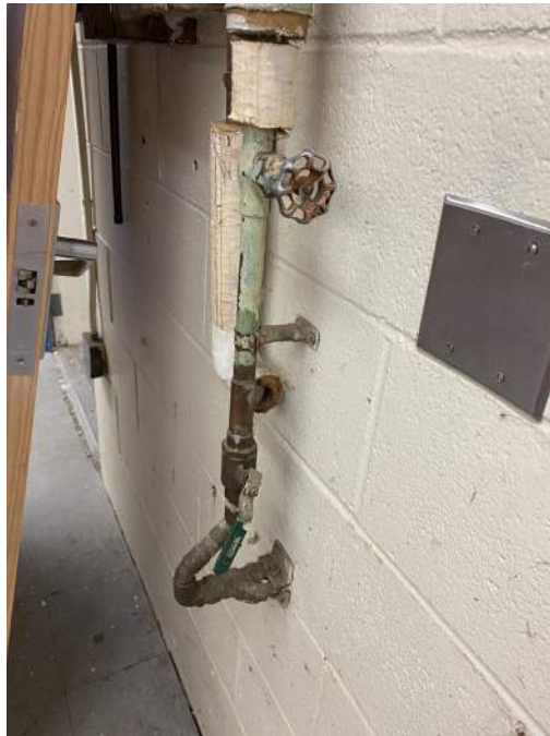
● D2. 9: Domestic Water Piping in Very Poor Condition.
