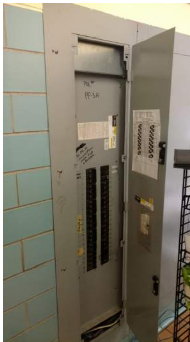
● D2. 15: Electrical Kitchen Branch Circuit Panel.
