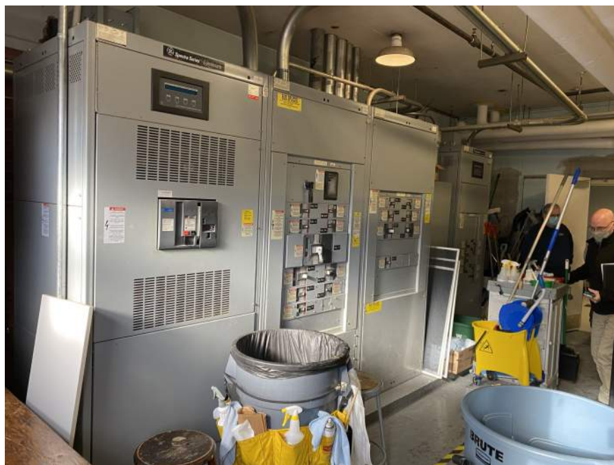
● D2. 16: Electrical Main Service Switchboard.
