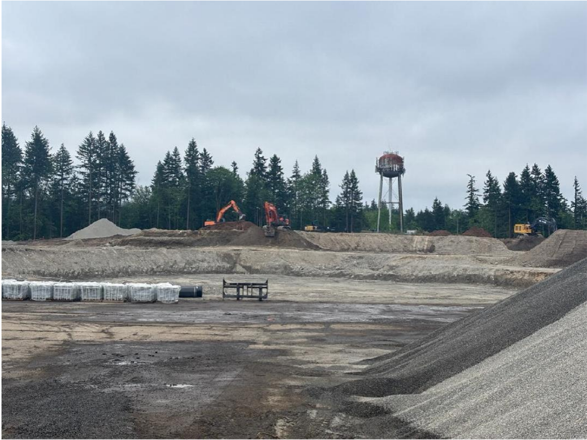
Excavation of the large storm pond that is located under the sports field
