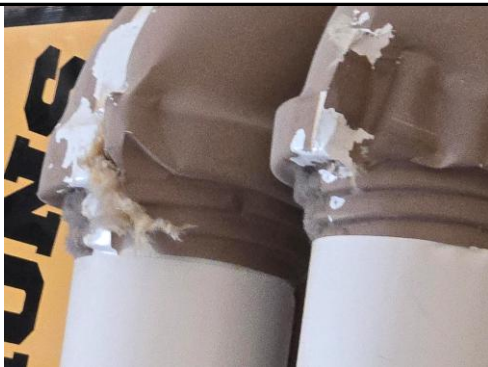
Pipe Insulation & Wrap
