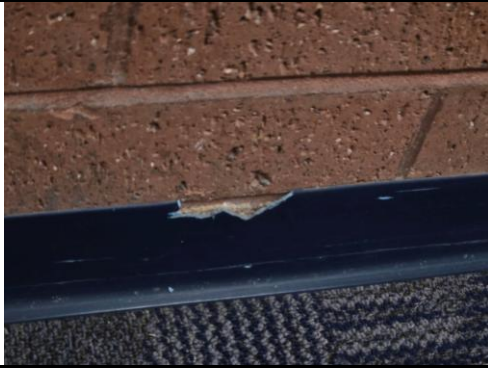
Black Stair Tread & Mastic
